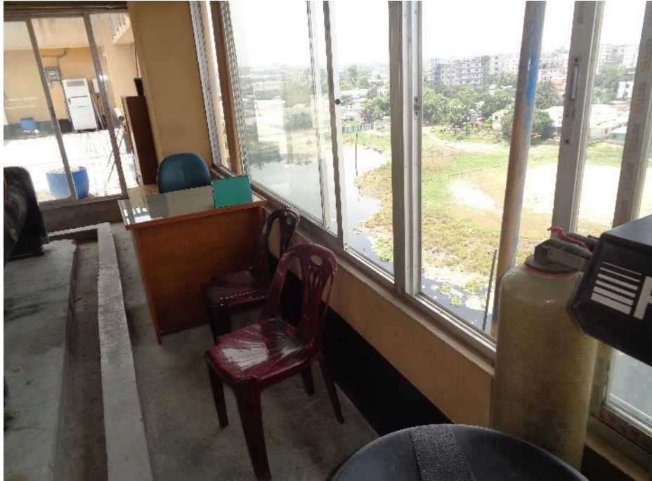
Low parapet height (700mm) at roof level
