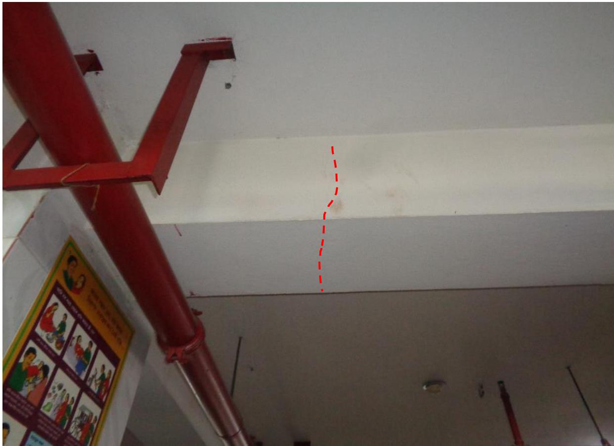
Hairline crack on beam under roof
