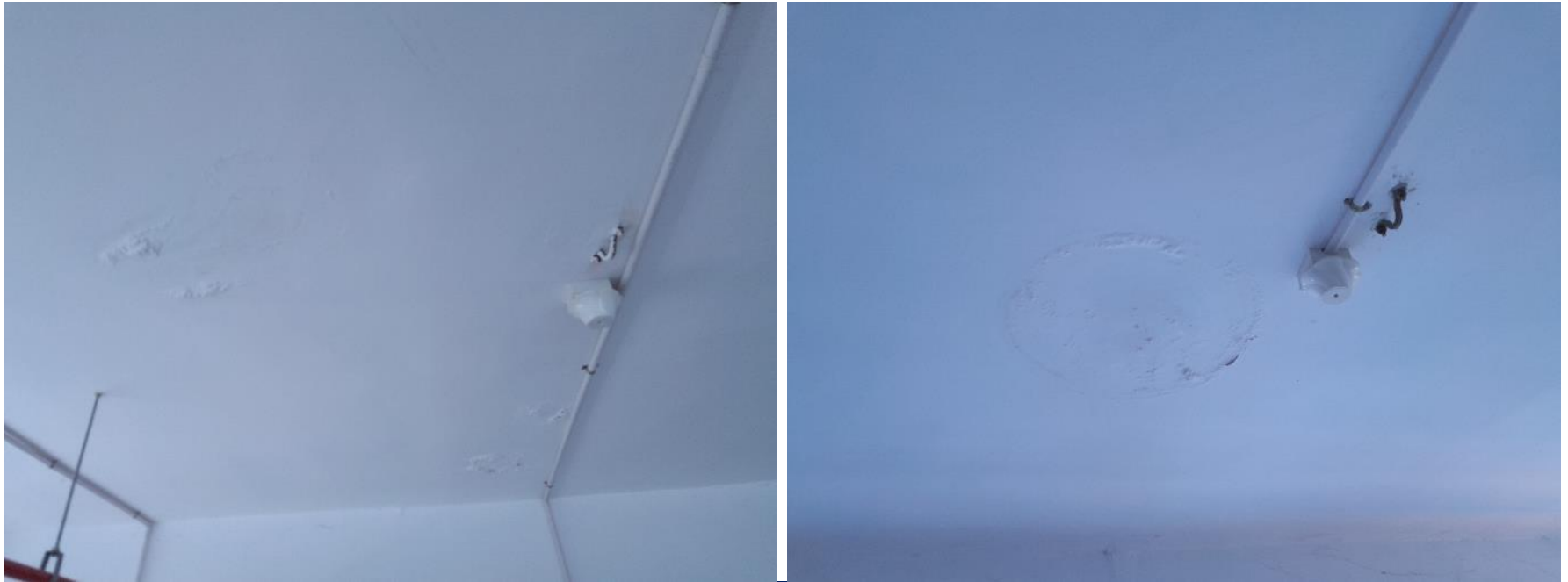
Dampness on slab soffit
