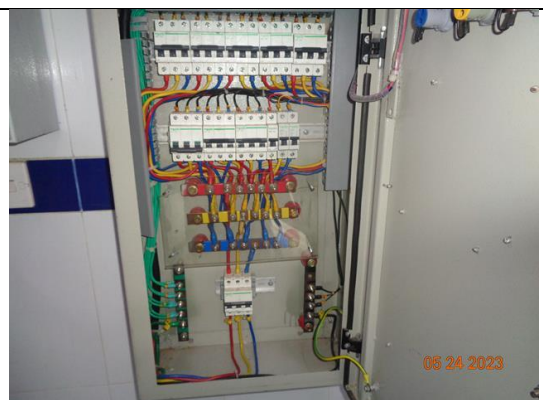
Typical Electrical Distribution Panel
