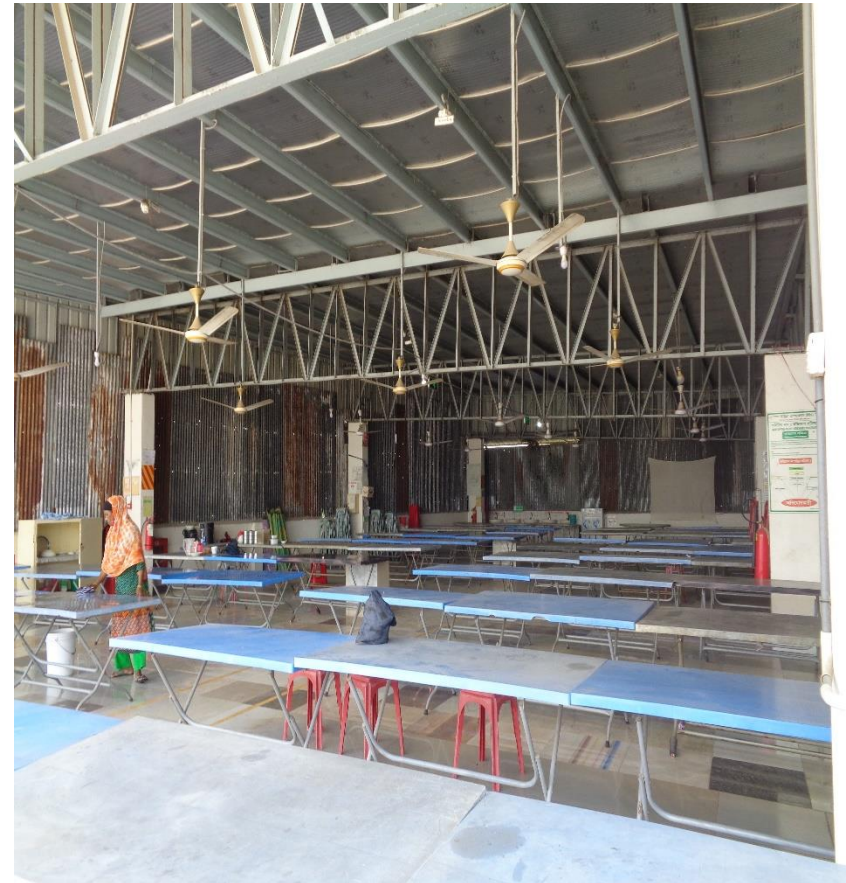
Truss frame and column not found on site
