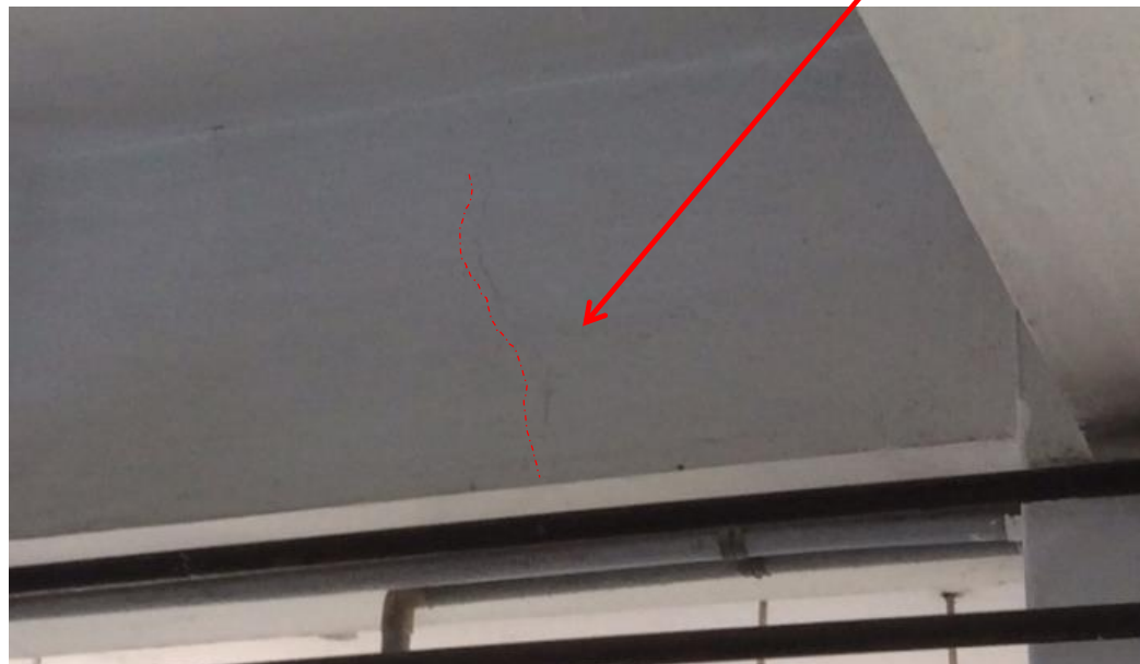
Cracking at beam ends
