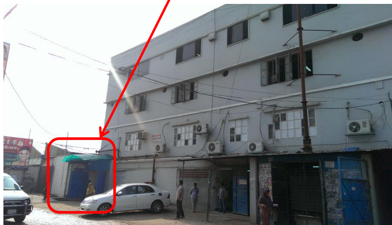
Non engineered steel roof
