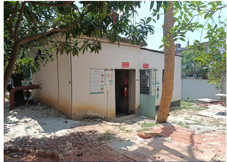
Fire Pump Room, ETP Shed
