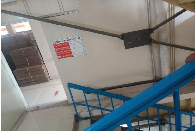
Incomplete bracing at the stair zone
