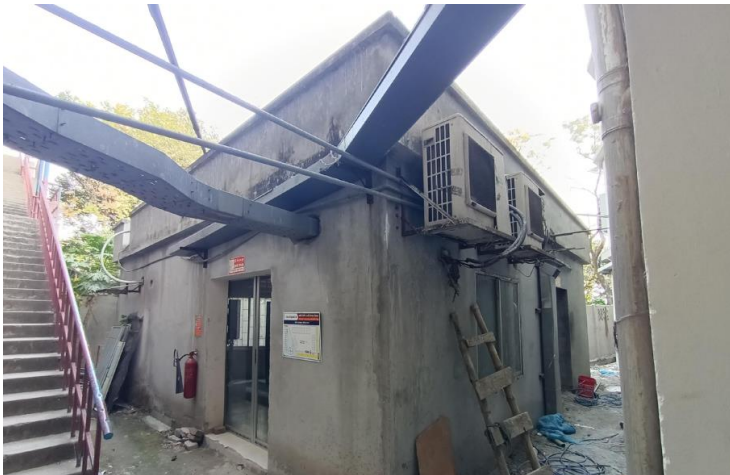
UPS & Compressor Room
