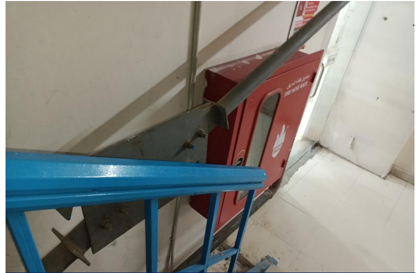
Incomplete bracing at the stair zone
