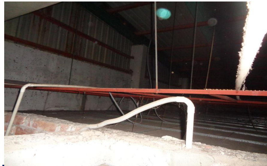
No tie beam in short direction at all grid
