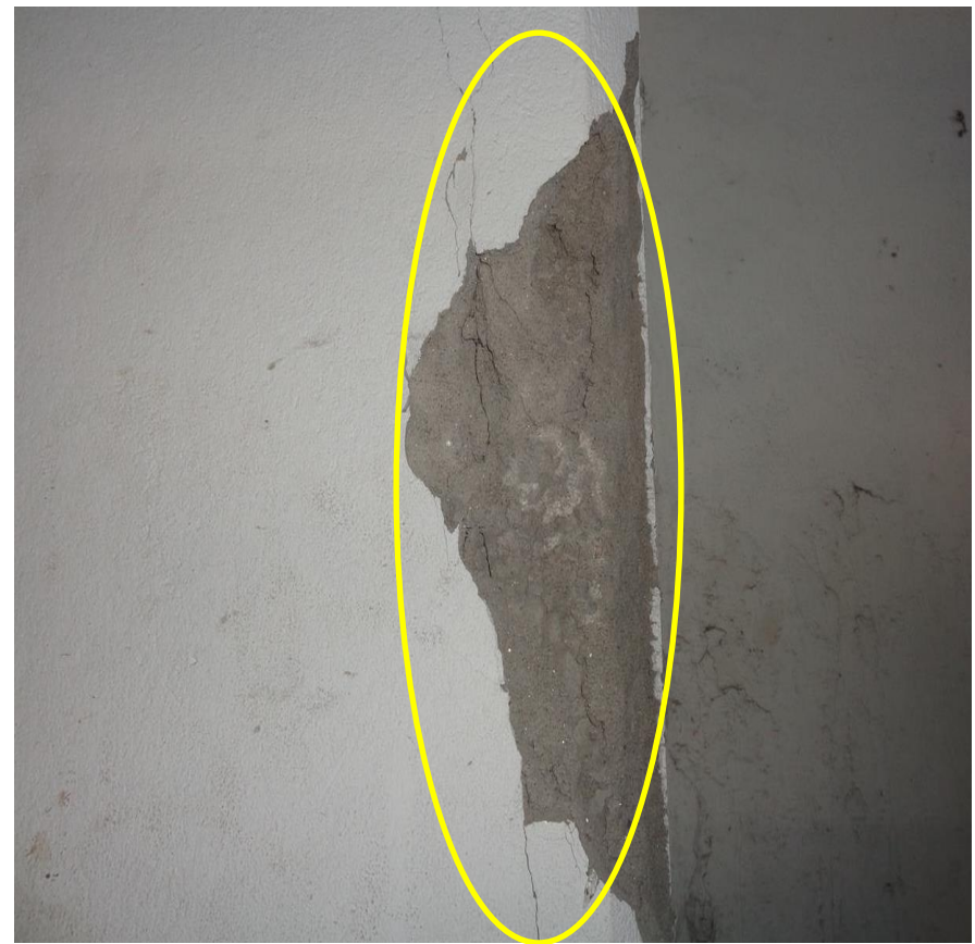
Crack on column surface
