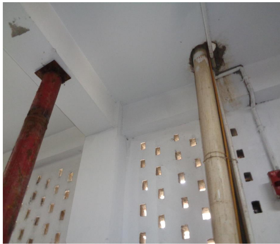
Crack on beam-column joint
