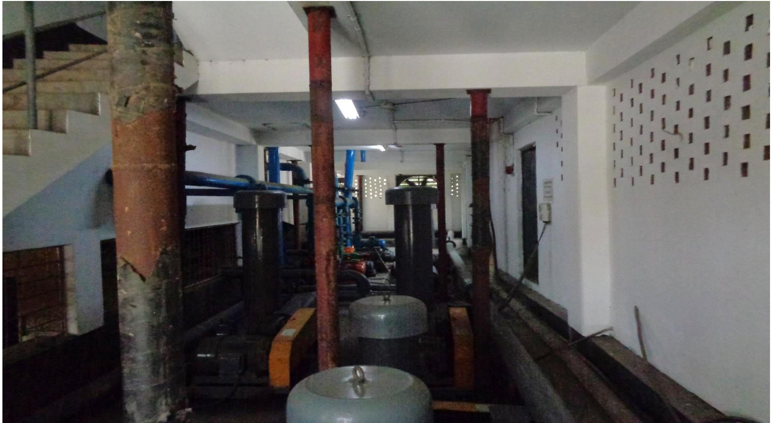
Heavy vibration at ground floor near blower machine
