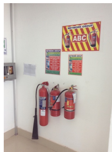
Dry chemical and CO fire extinguisher
