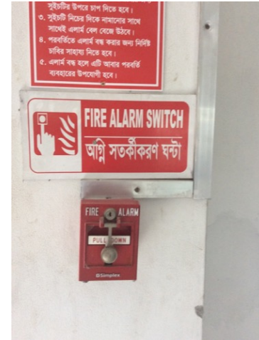
Manual pull alarm
