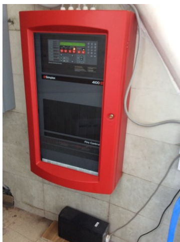
Fire alarm panel
