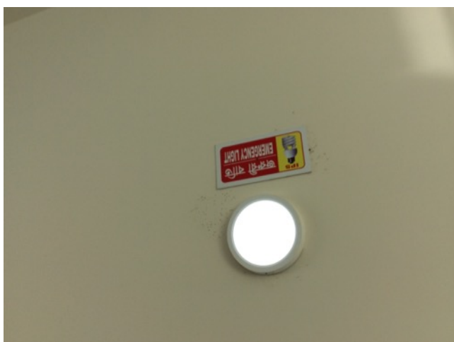
IPS powered emergency light
