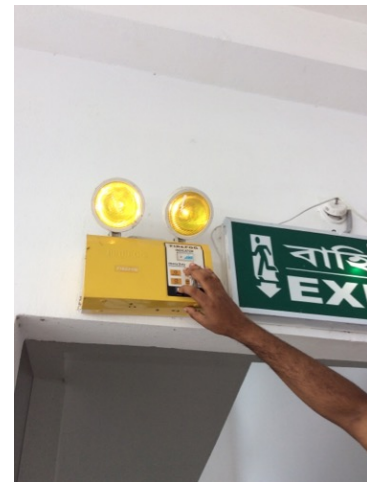
Exit sign and emergency light
