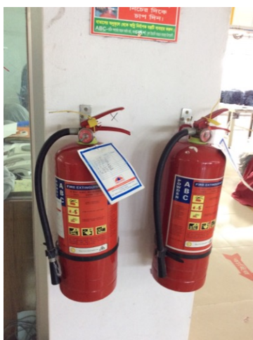
Dry chemical extinguisher
