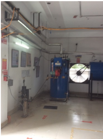
Gas fired boiler
