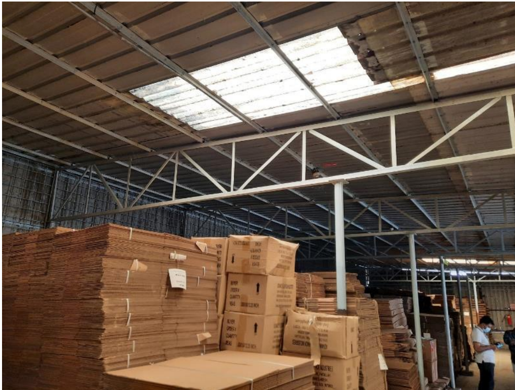
No roof & wall bracing provided
