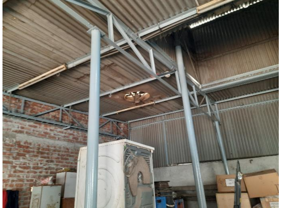
Column support out of node
