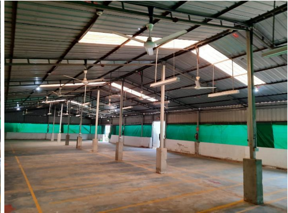
No roof & wall bracing provided
