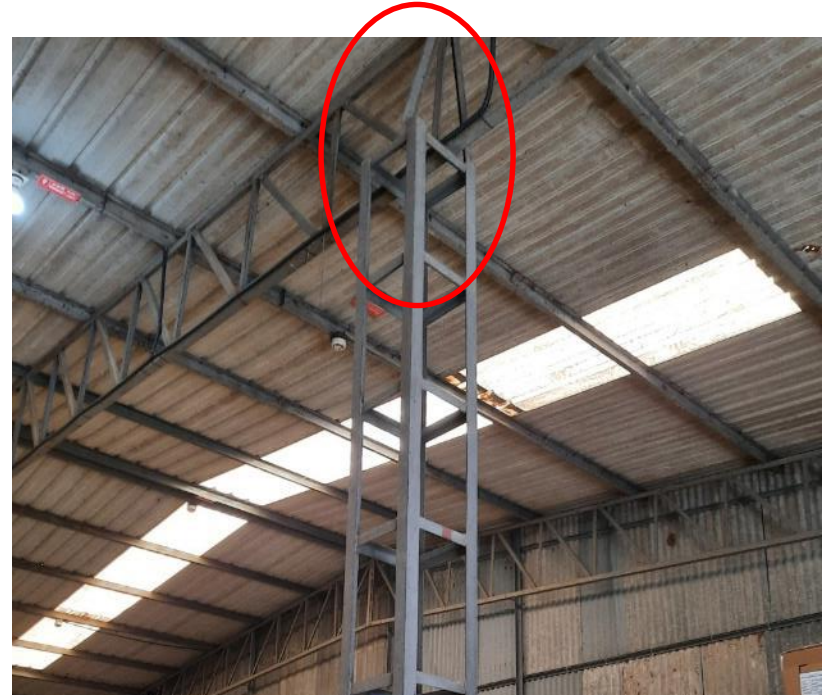
Poor connection system
