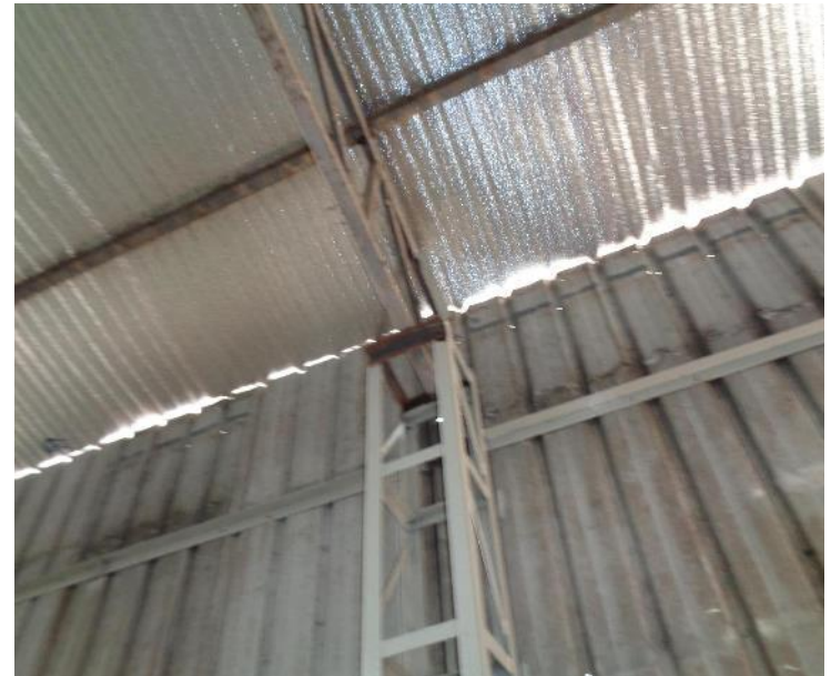
Poor connection system
