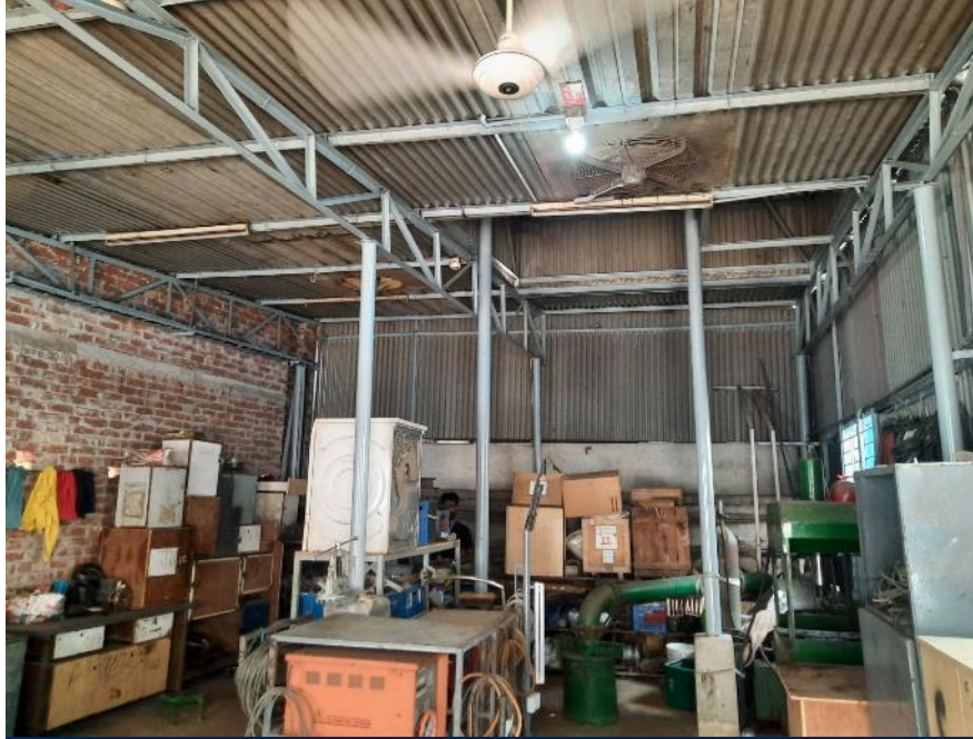
No roof & wall bracing provided
