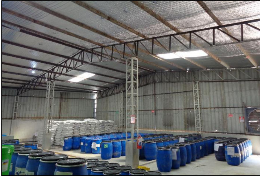
No roof & wall bracing provided
