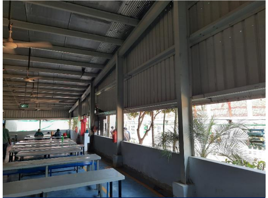
No roof & wall bracing provided
