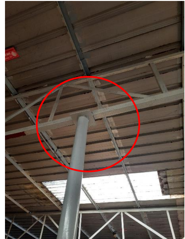
Poor connection system
