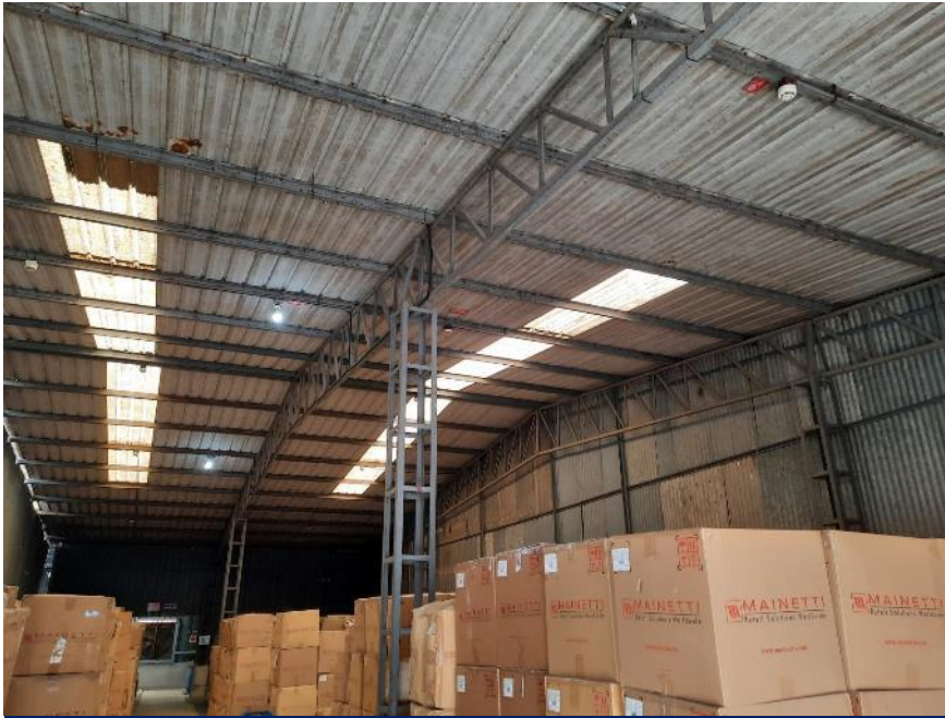
No roof & wall bracing provided
