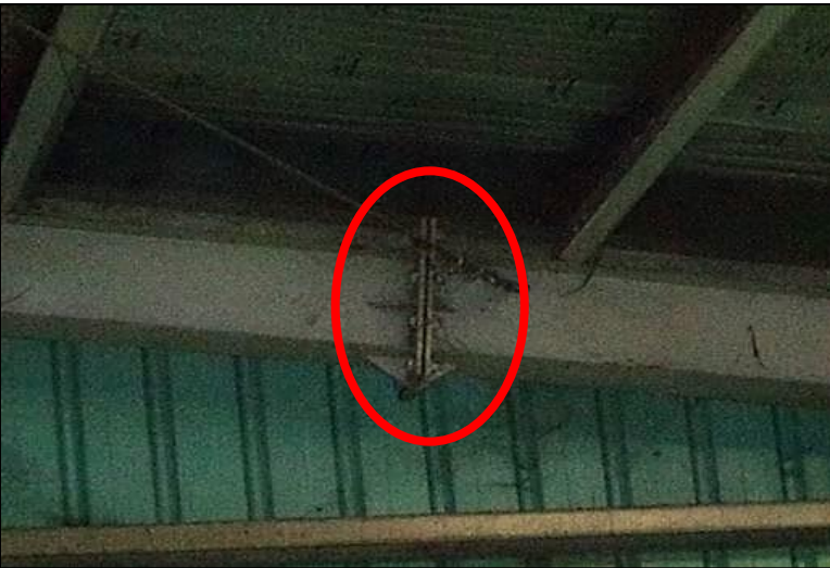
Significant connection gap
