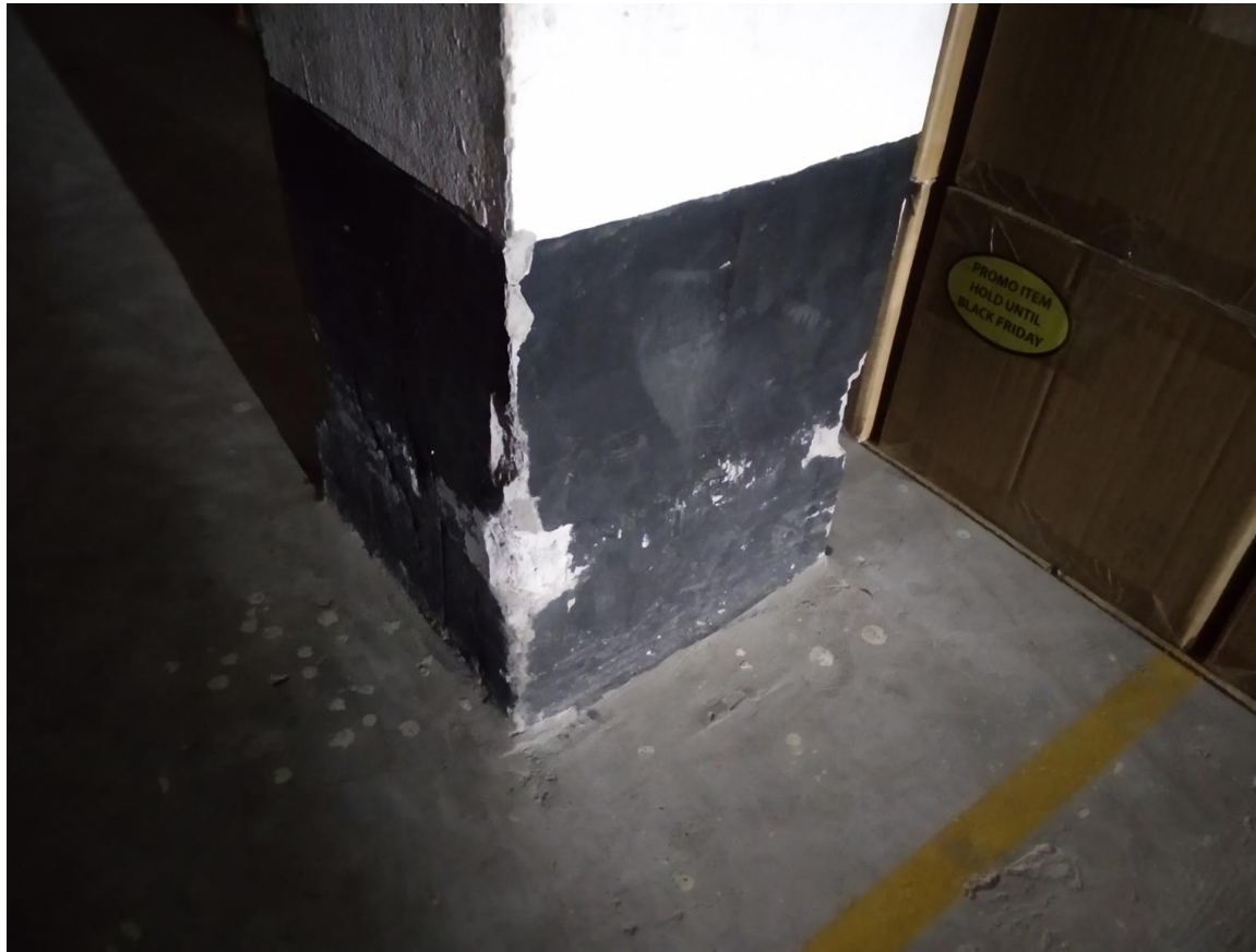
Column damaged by the trolley movement
