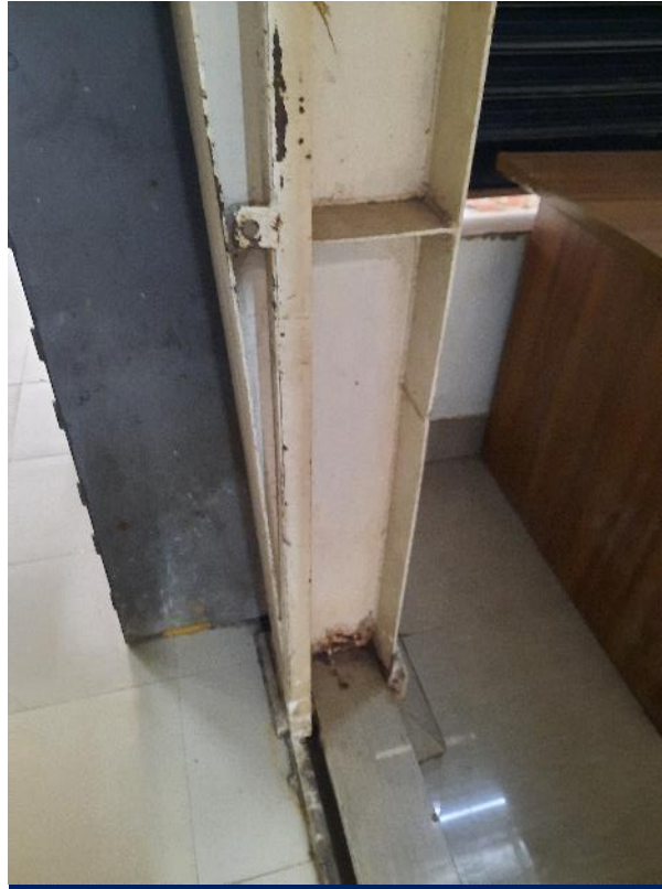
Corrosion (Dinning ware house)
