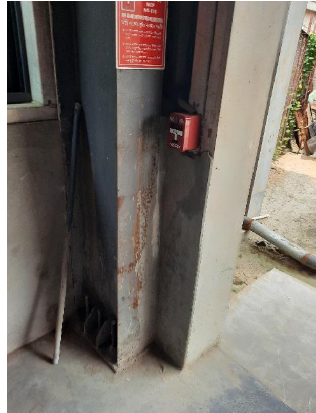
Corrosion (Fire pump room)
