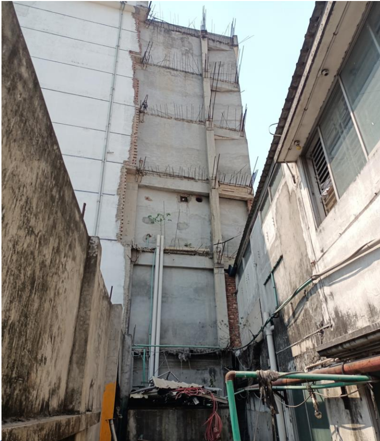
Corrosion at exposed rebar
