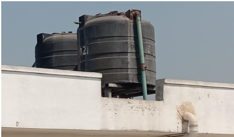
Plastic water tank not braced
