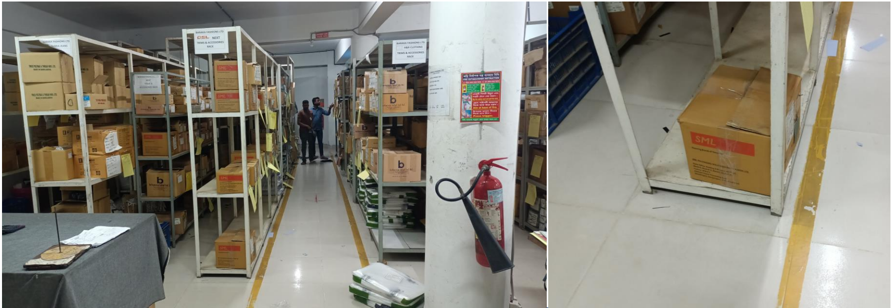
Non-anchored storage rack at several floors
