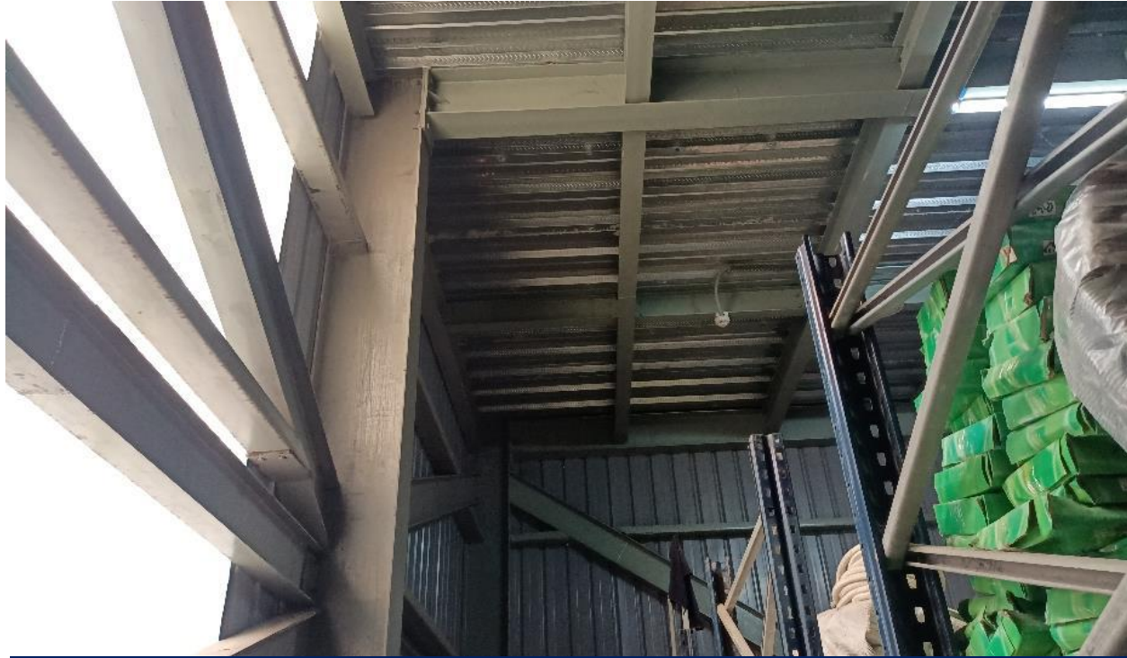
Inside of EGB Room
