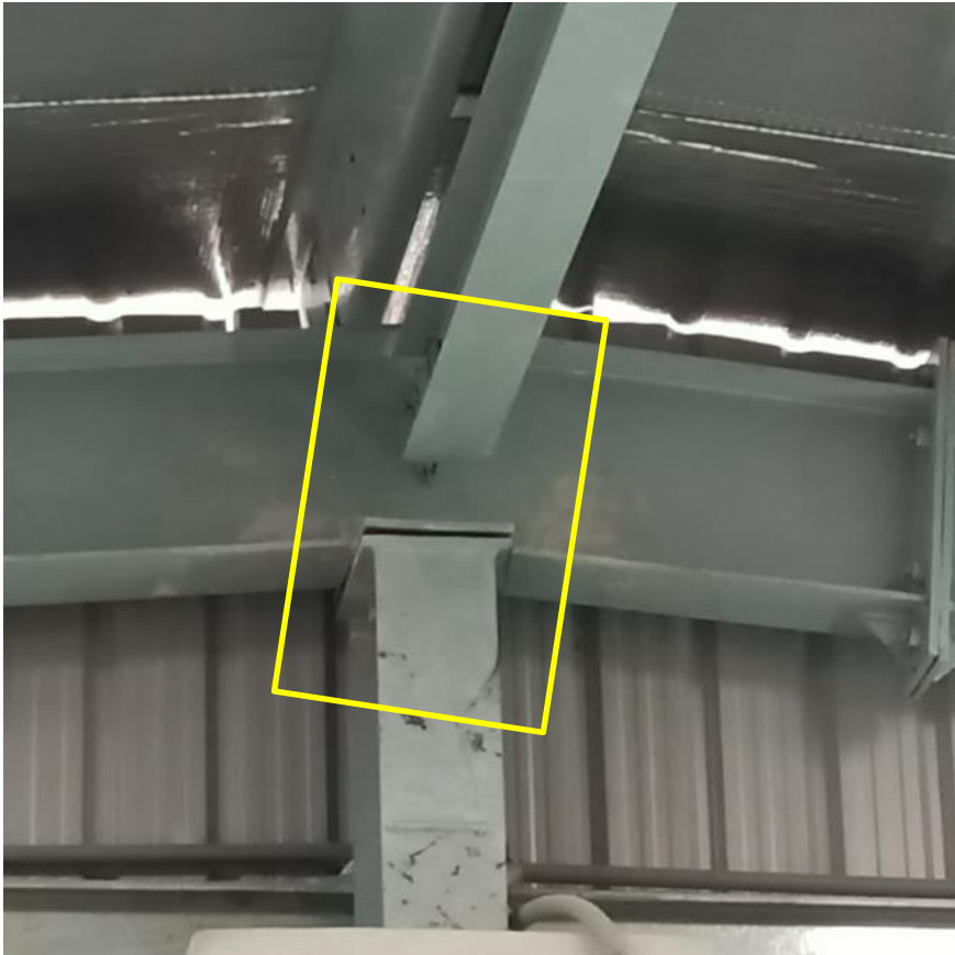
Gap observed in connections
