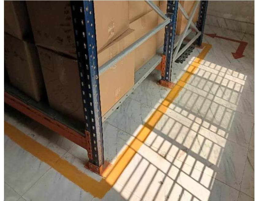
Racks without anchoring
