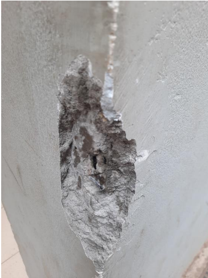
Stone chips aggregate on column
