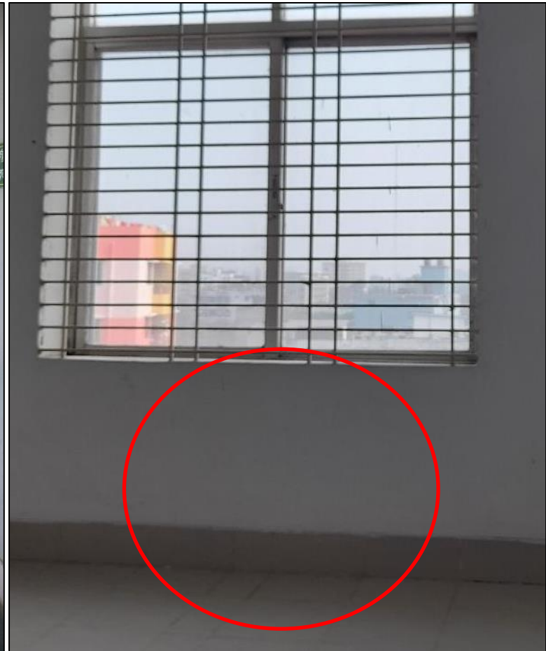
Dampness due to water ingress
