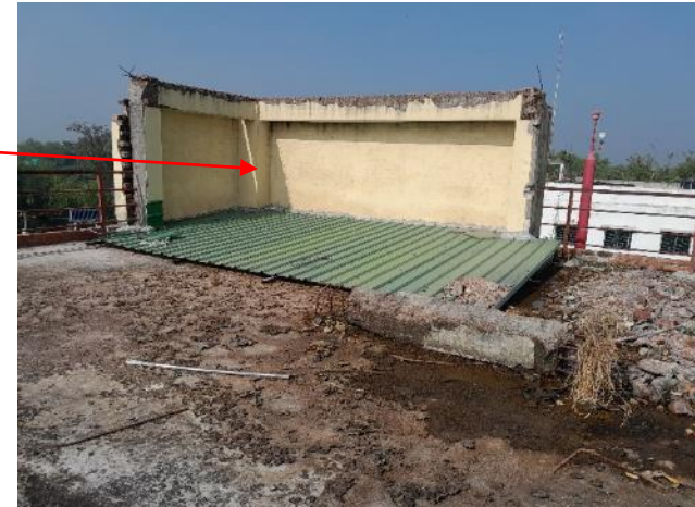
Stair was found demolished.
