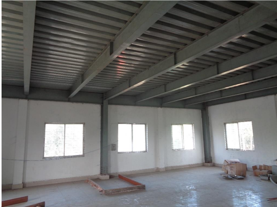
Additional plate not installed in steel beam
