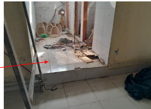
200 mm build up found at toilet
