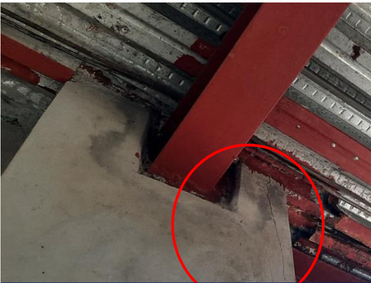
Crack on RC column and steel beam joint
