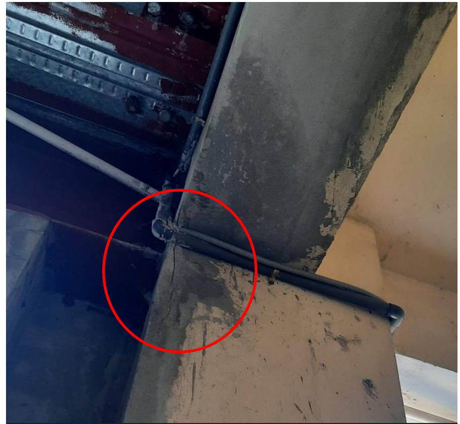
Crack on RC column and steel beam joint
