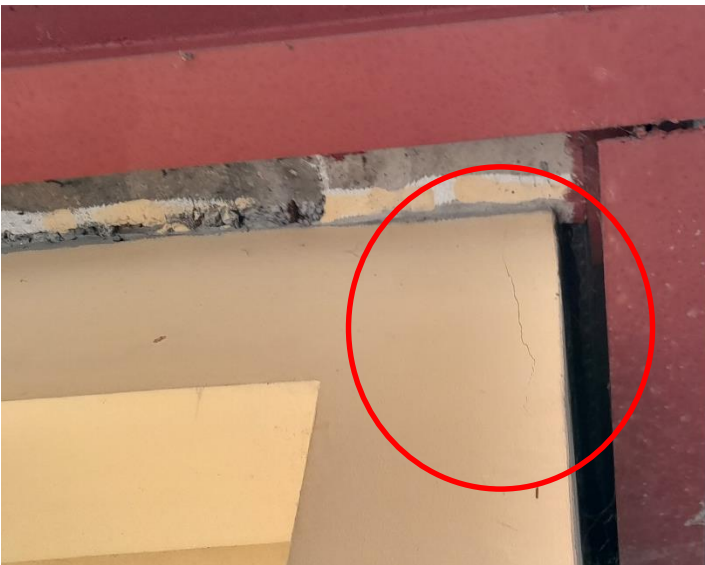
Crack on RC beam-column joint
