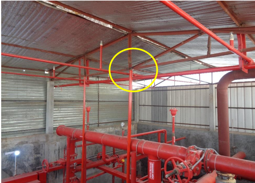
No joint plate observed in truss to column joint
