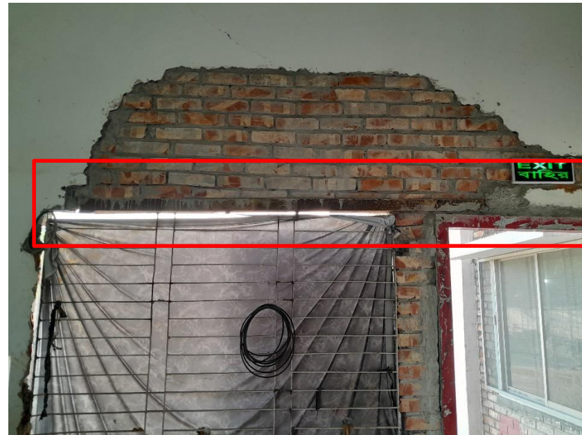
Corroded and deflected steel member support instead of lintel
