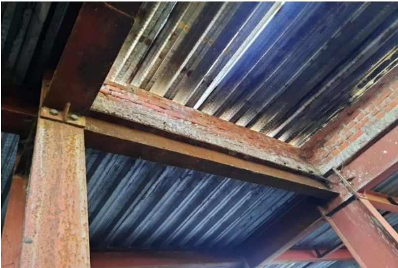
Severe corrosion on steel members
