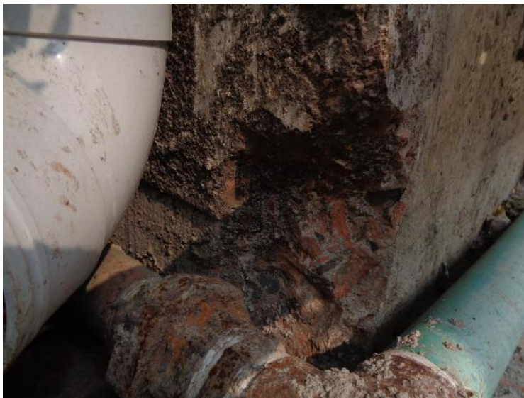
Brick aggregate in column of Building-4
