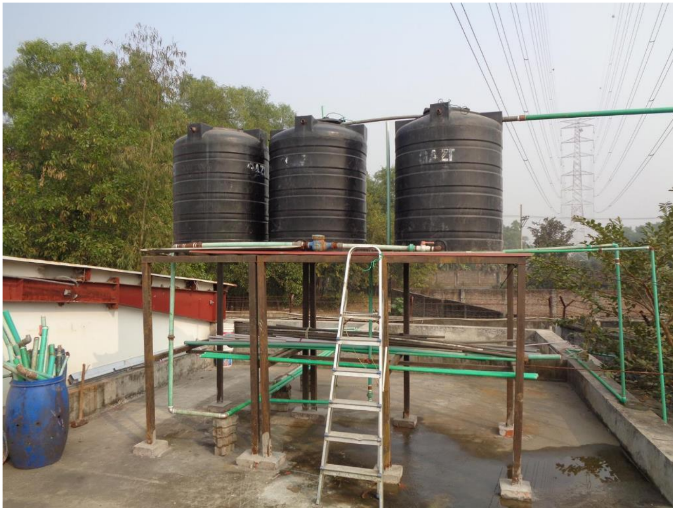
Unbraced plastic water tanks on roof
