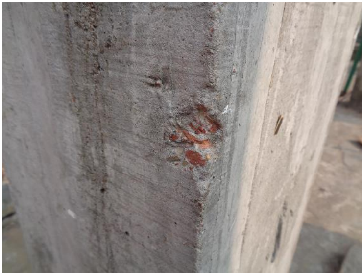
Brick aggregate in column of Building-13
