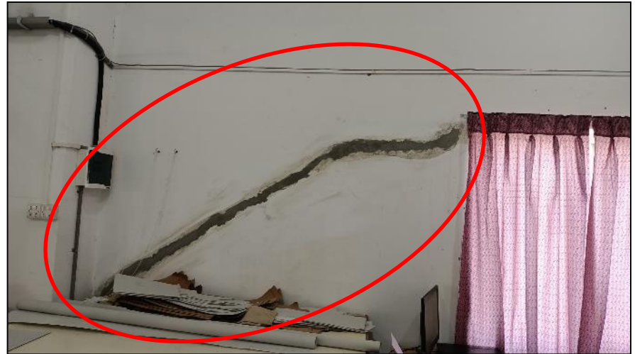
Crack at 5 th floor
