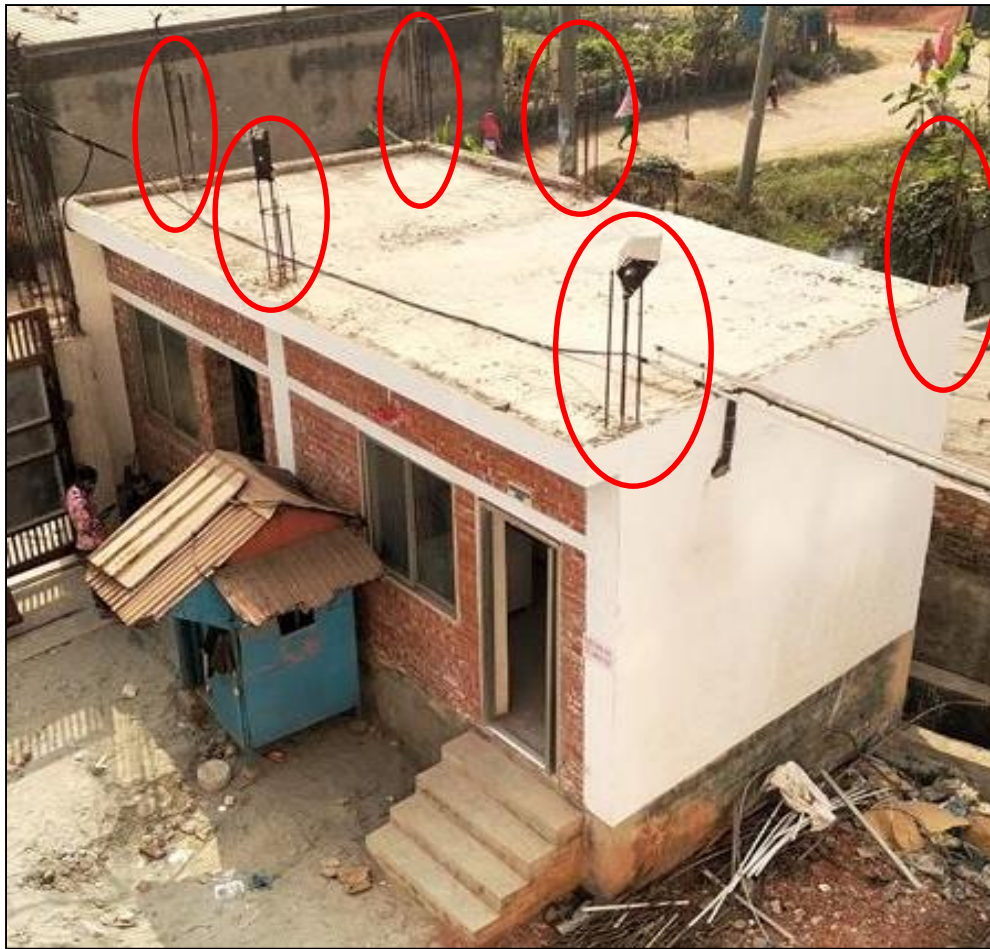
Exposed rebar at rooftop
