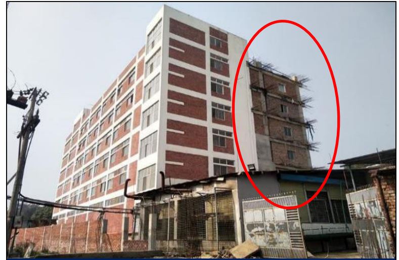
Exposed rebar at east side
