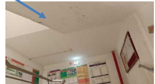
Missing beam at stair landing
