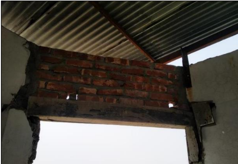
Inadequate lintel support at RO plant at roof level
