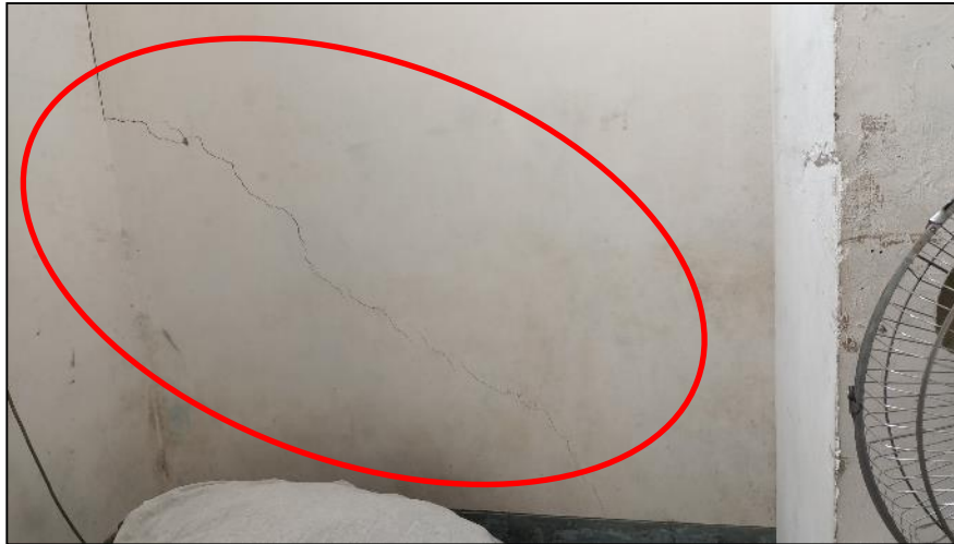
Crack at ground floor
