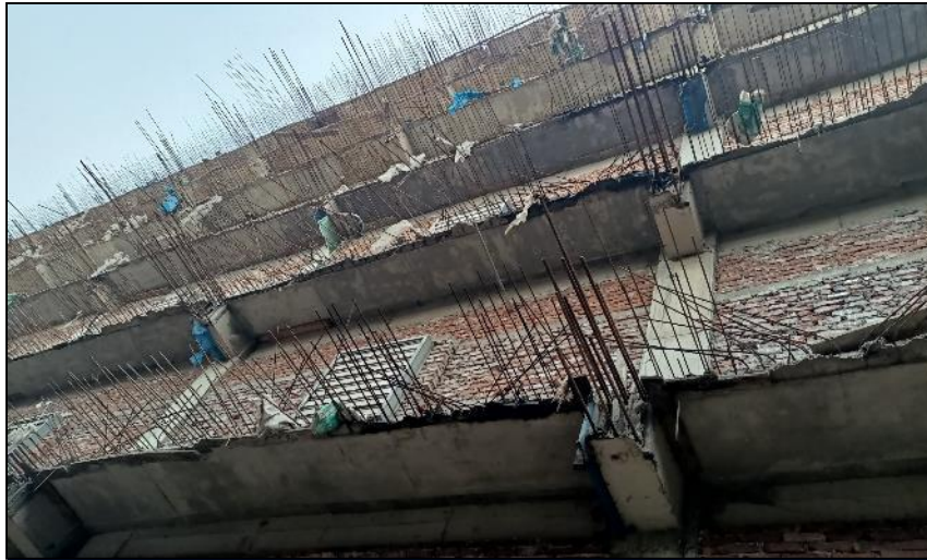
Exposed rebar at north side
