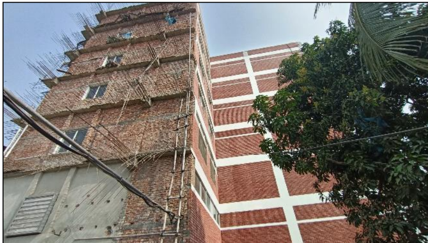
Exposed rebar at west side
