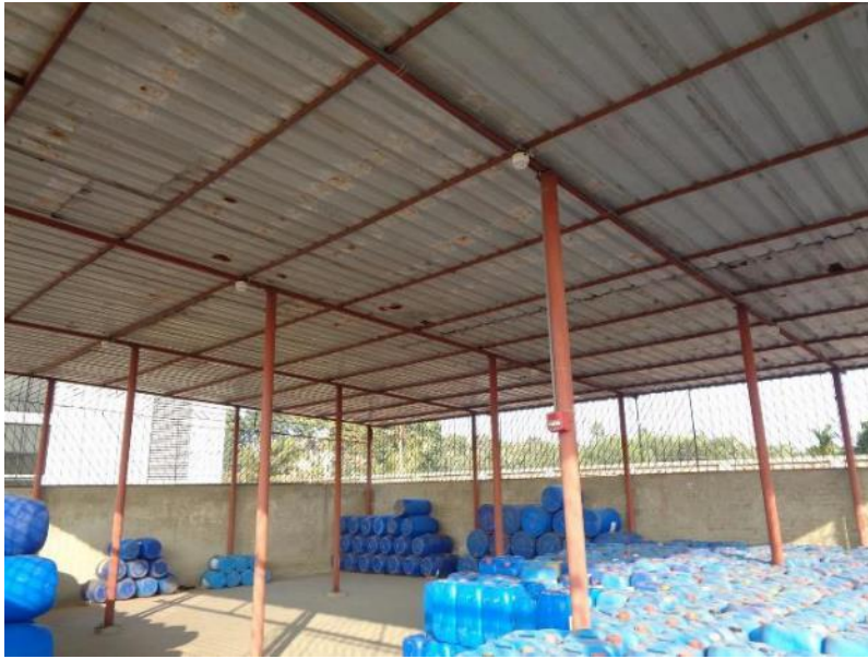
Lateral load resisting system (bracing, compression strut) is absent
