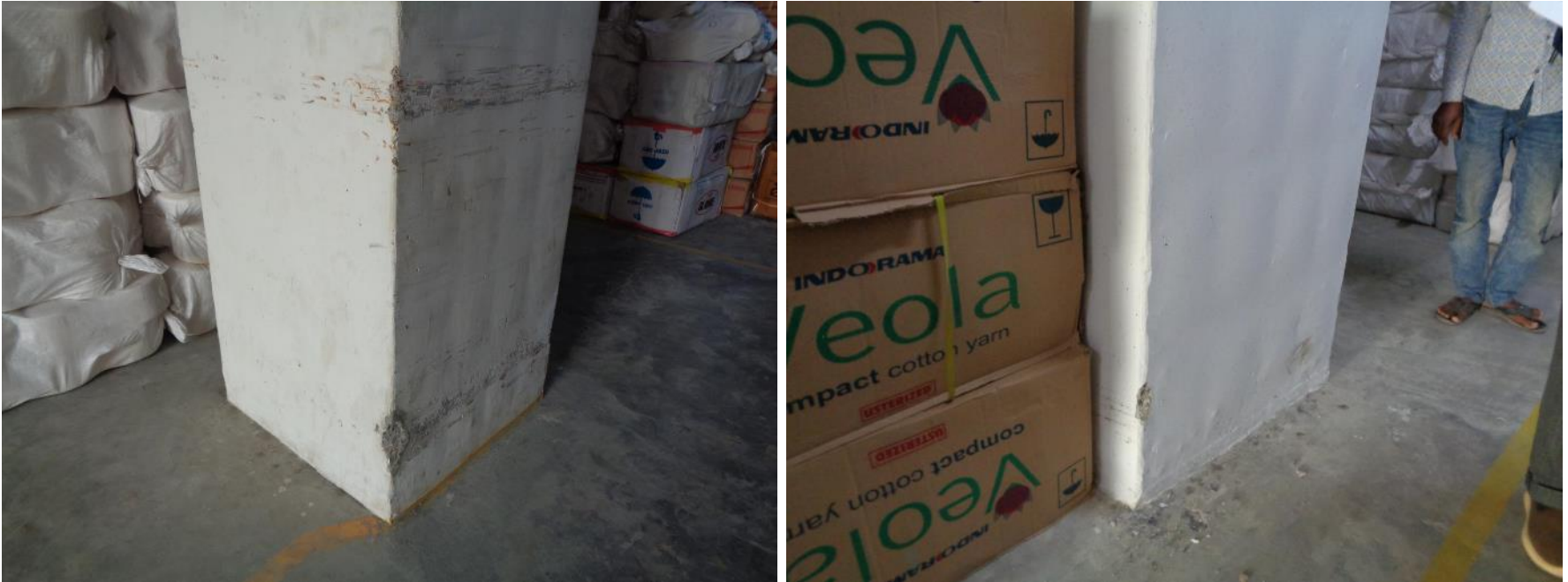
Column damage due to trolley impact
