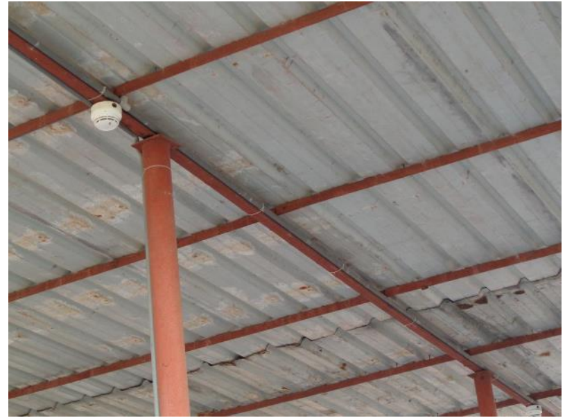
Apparently inadequate connections (minimum size of welding)
