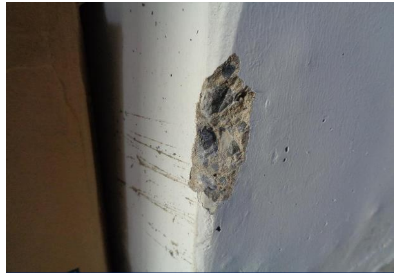
Brick aggregate in column of Building-16
