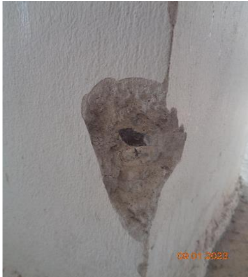
Stone aggregate in column of Building-17
