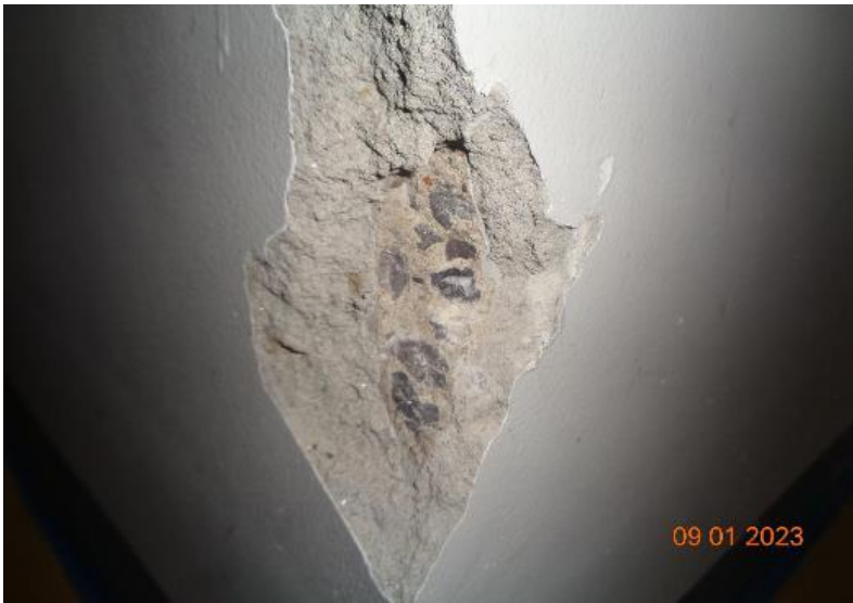
Stone aggregate in column of Building-15
