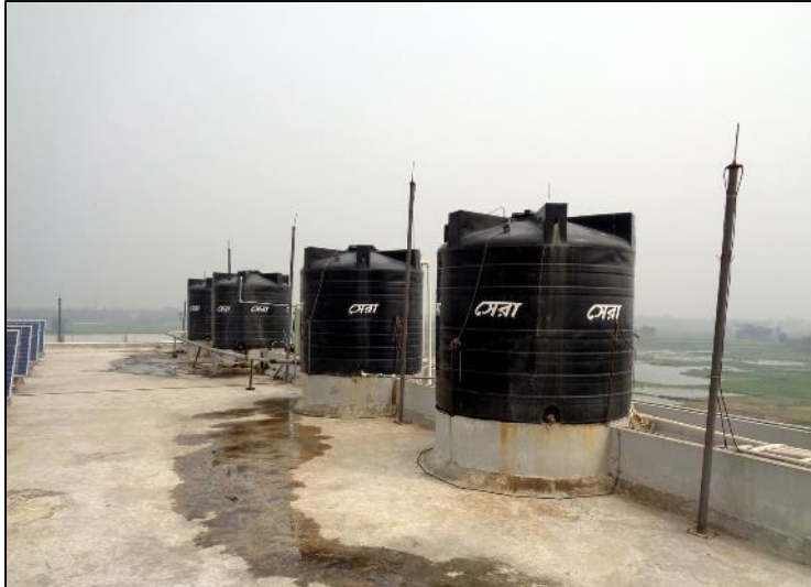
Water tank location in the roof
