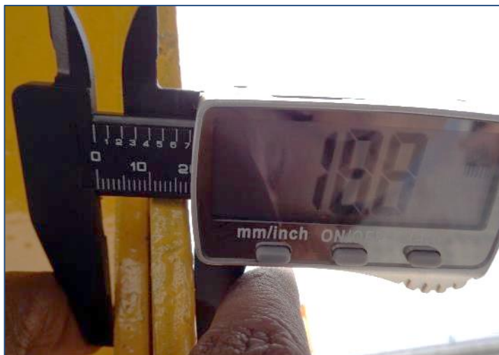
Flange thickness in C-209 column found 18 mm (double plate) instead of 10 mm (single plate)
