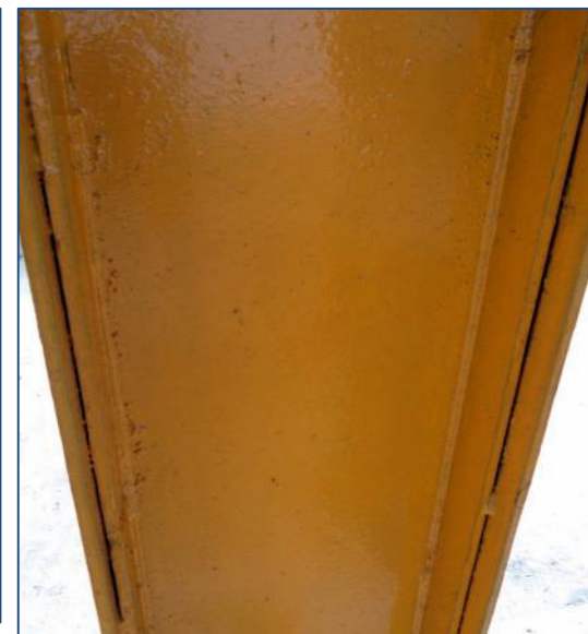
Additional plate was found in the C-209 steel column
