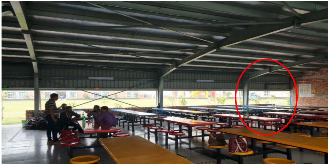
Bracing missing this marked location
