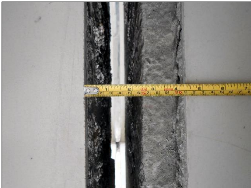
Expansion gap with 2.5 inch was found on 3 rd and 4 th floor
