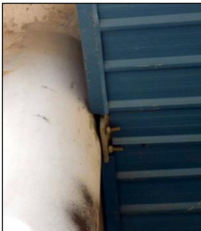
Gap in the Connection to column
