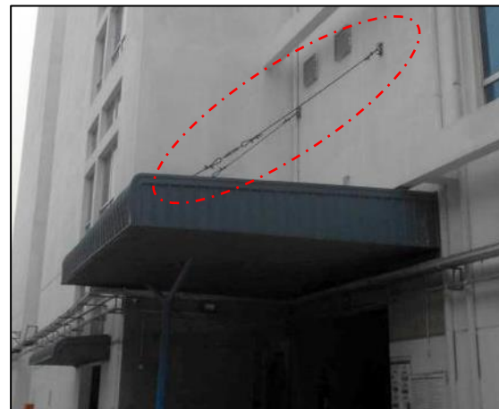
Cable Connection to wall
