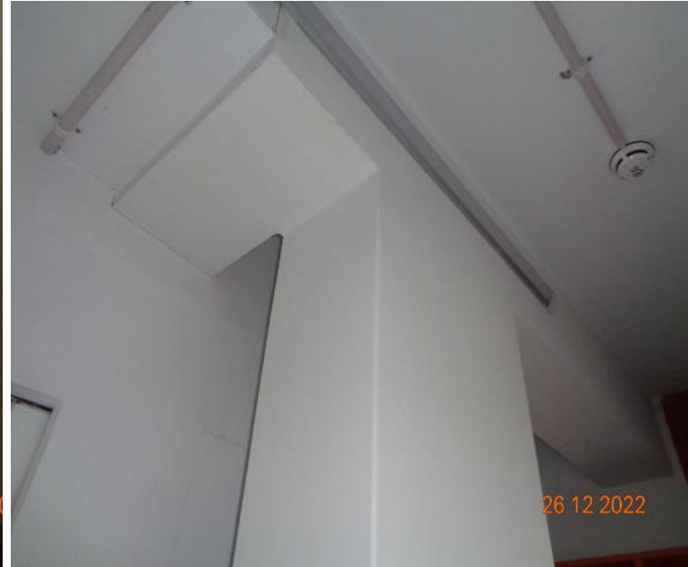
Large offset of beam from column line
