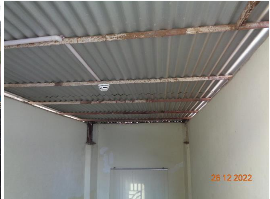
Lack of anchorage between roof and columns
