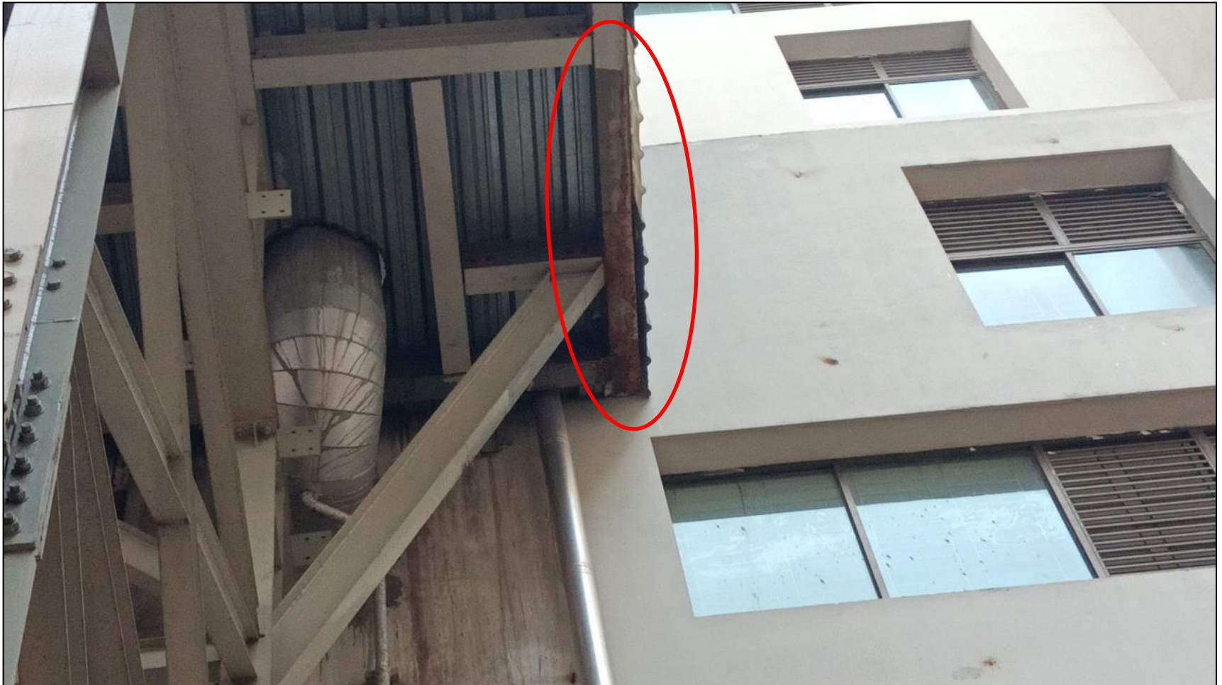
Corrosion in cantilever steel beam
