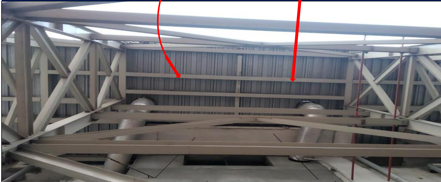
Some sub-beam found missing at on-site
