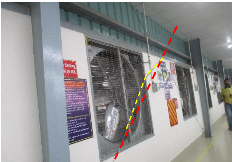
Improper loose wall bracing
