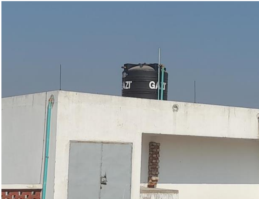
Plastic water tank on roof
