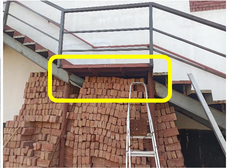
Inadequate support and discontinue beam
