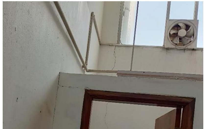
Cracks on brick wall on ground floor
