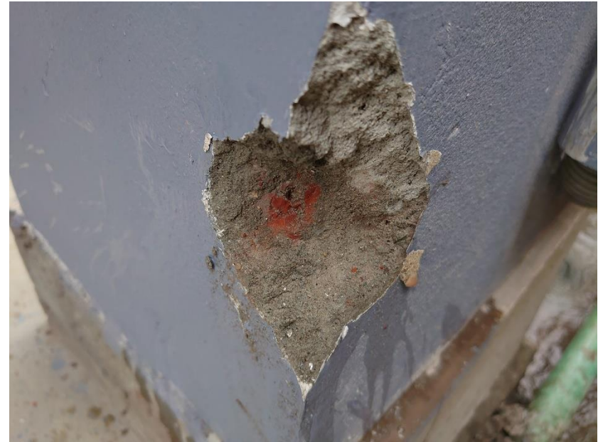
Brick chips found as aggregate in columns
