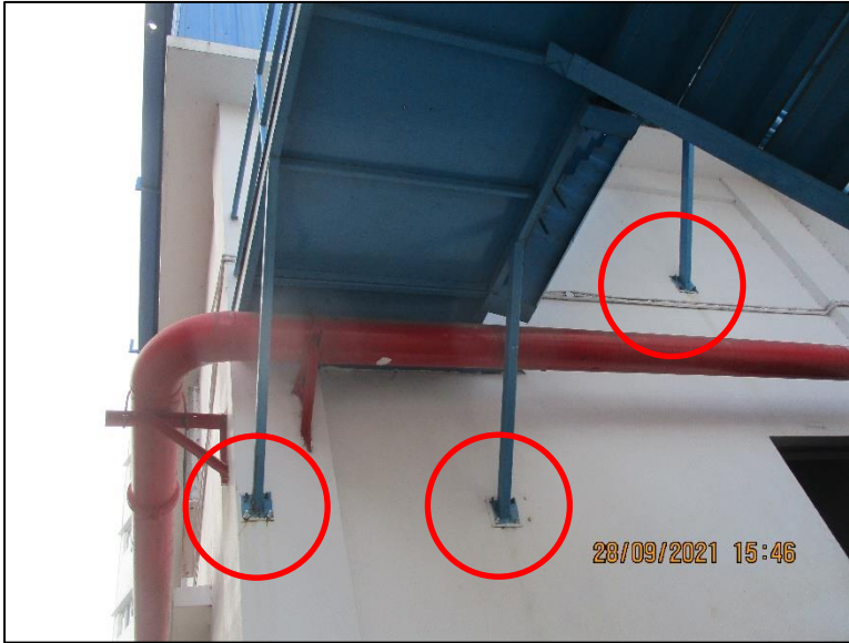
Apparently Inadequate Connection
