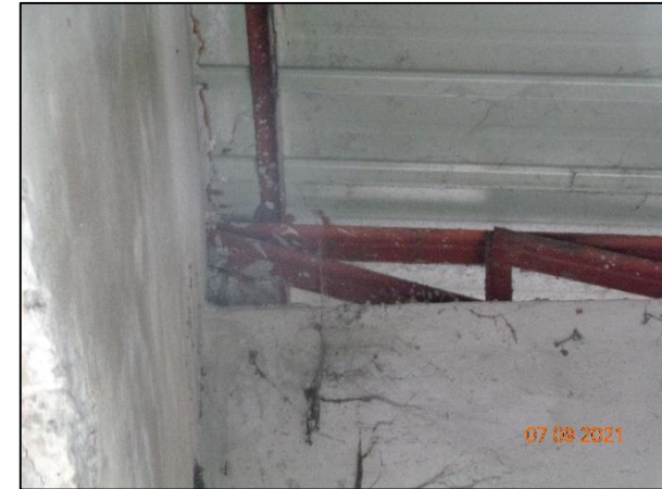
Poor connection details
