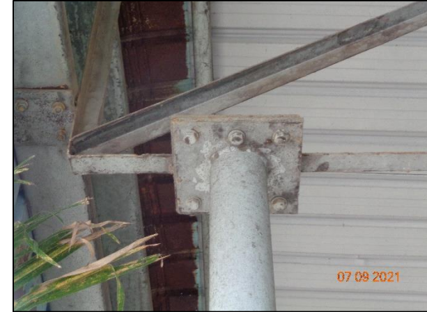
Poor connection details
