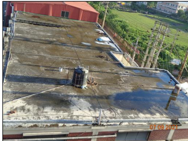
Water ponding at roof
