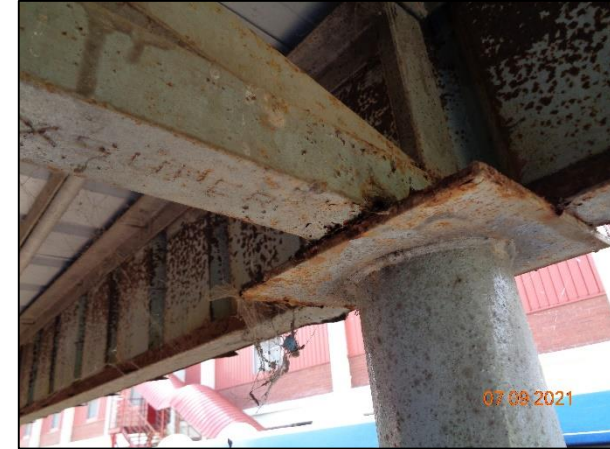
Poor connection details
