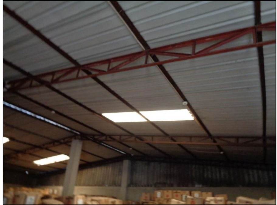
Lack of lateral bracing
