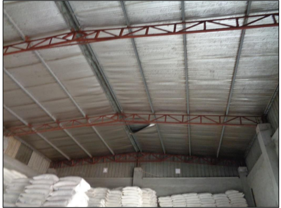
Lack of lateral bracing
