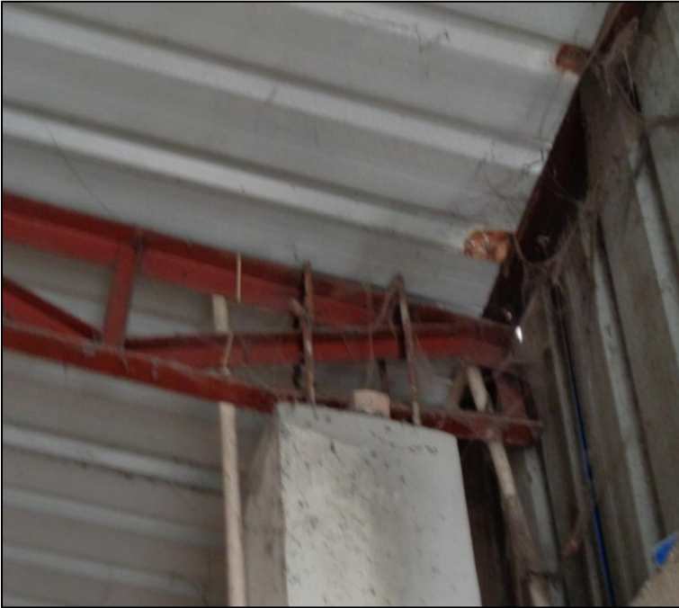
Poor connection details
