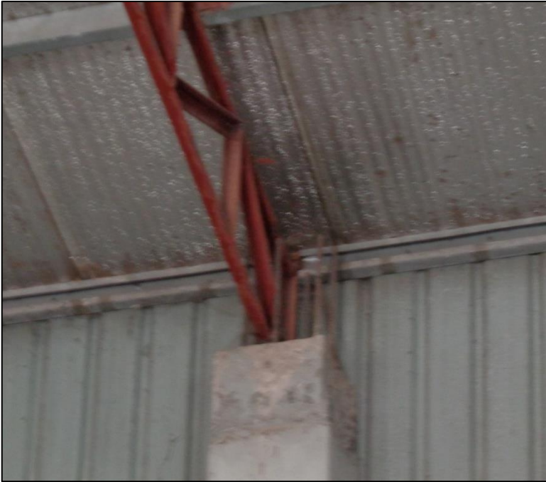
Poor connection details
