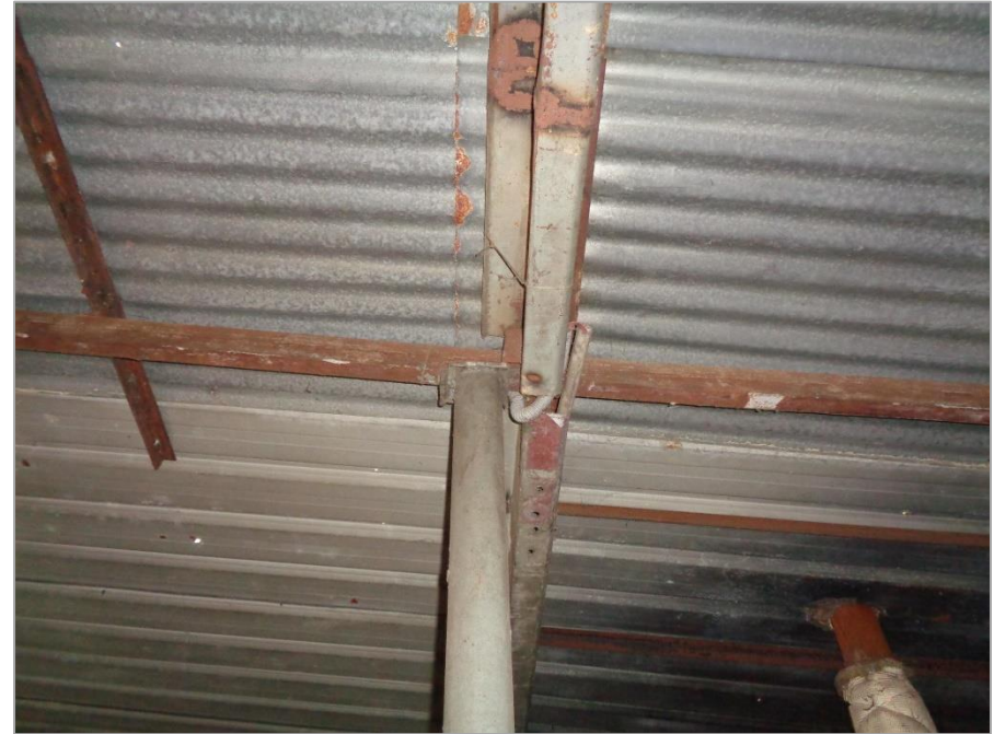
Non engineered connection
