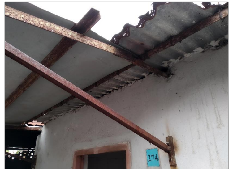
Non engineered connection
