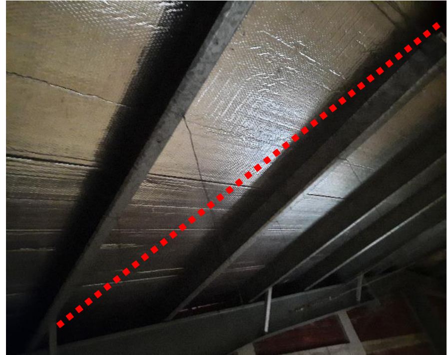
Missing roof bracing
