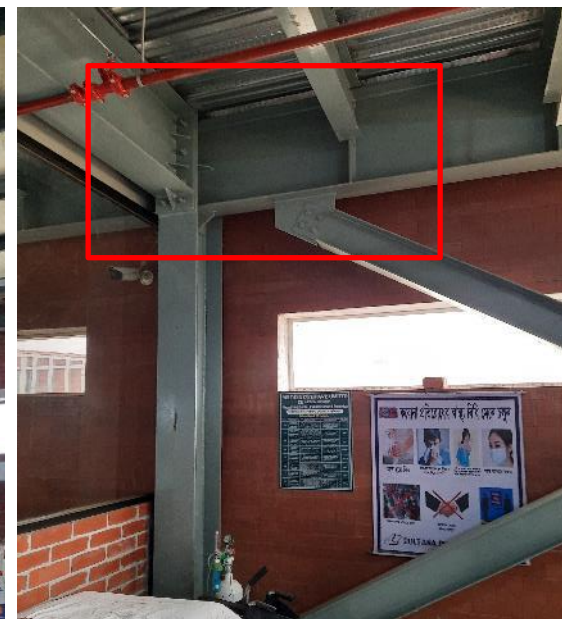
Bracings are offset from the node point- Shed 5
