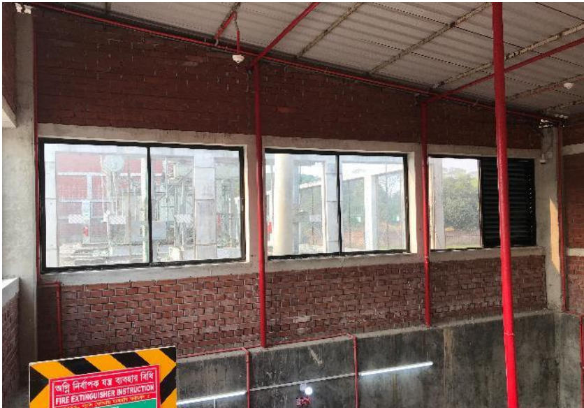
Inadequate structural members
