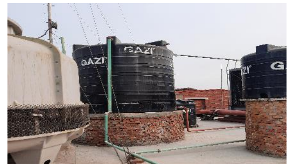
Water tank with build-up
