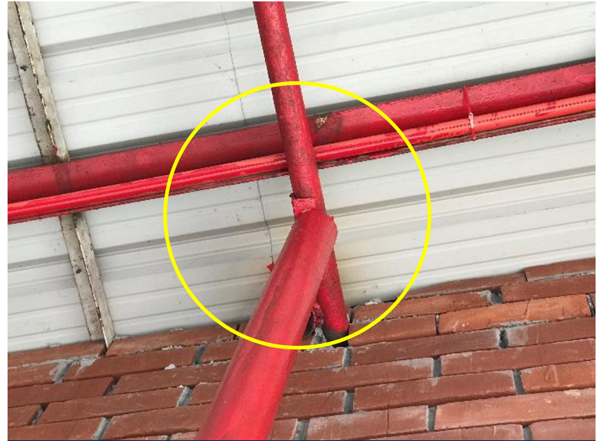
Poor connection details
