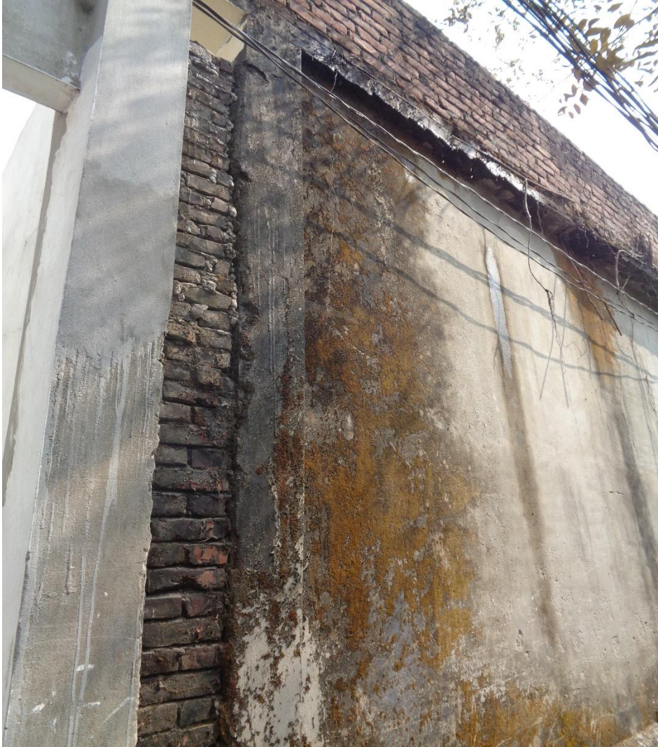
Severed dampness was found in façade at west side
