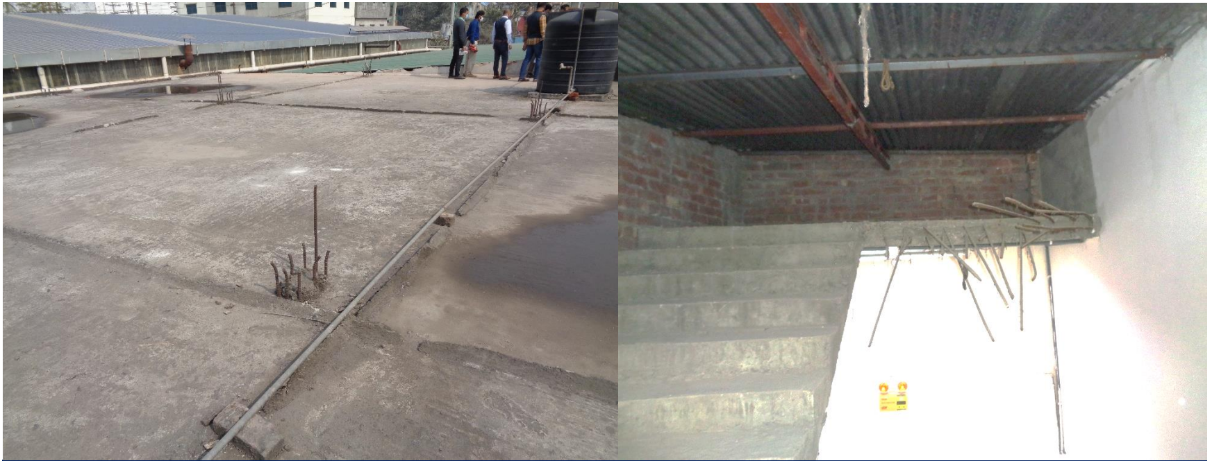
Exposed reinforcement left at roof level & staircase.
