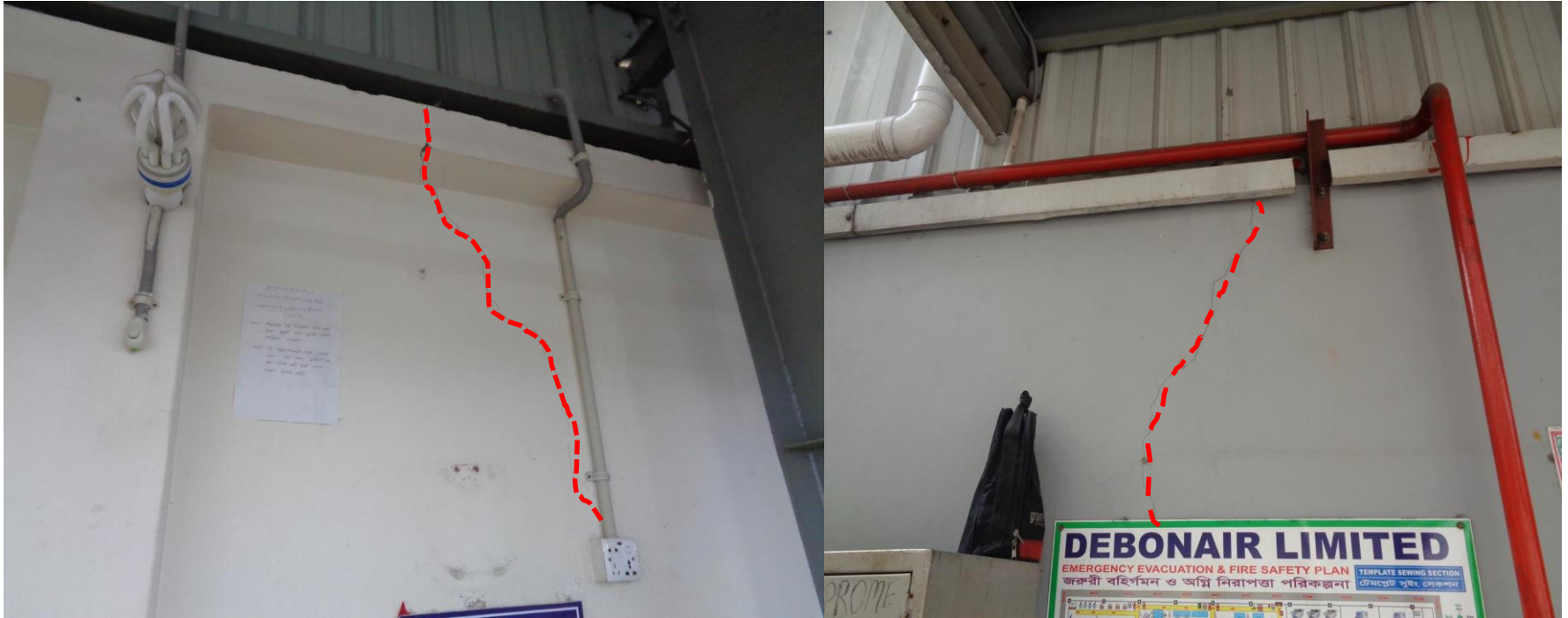
Crack in brick wall
