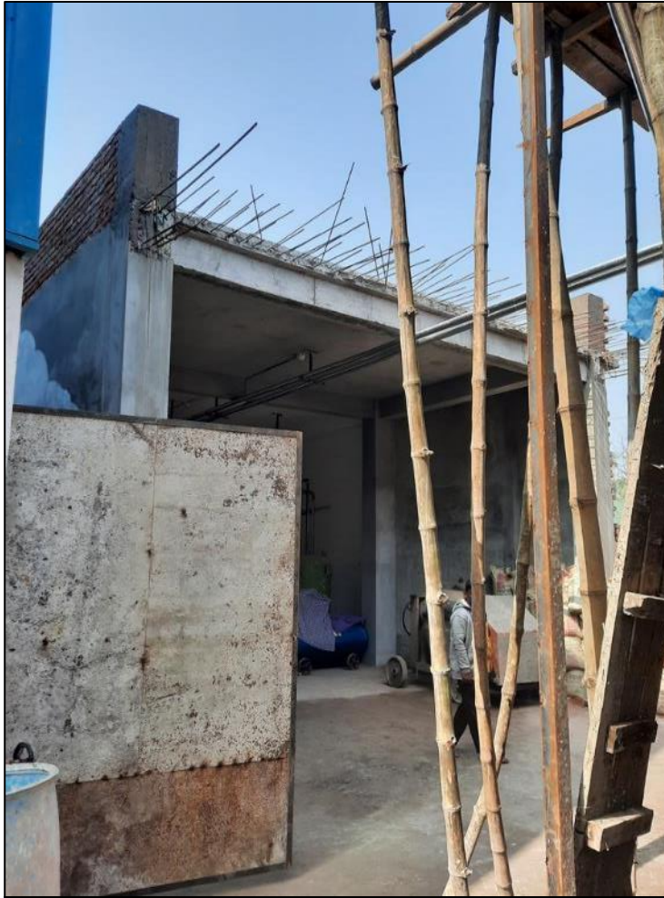
Exposed rebar of beam and slab
