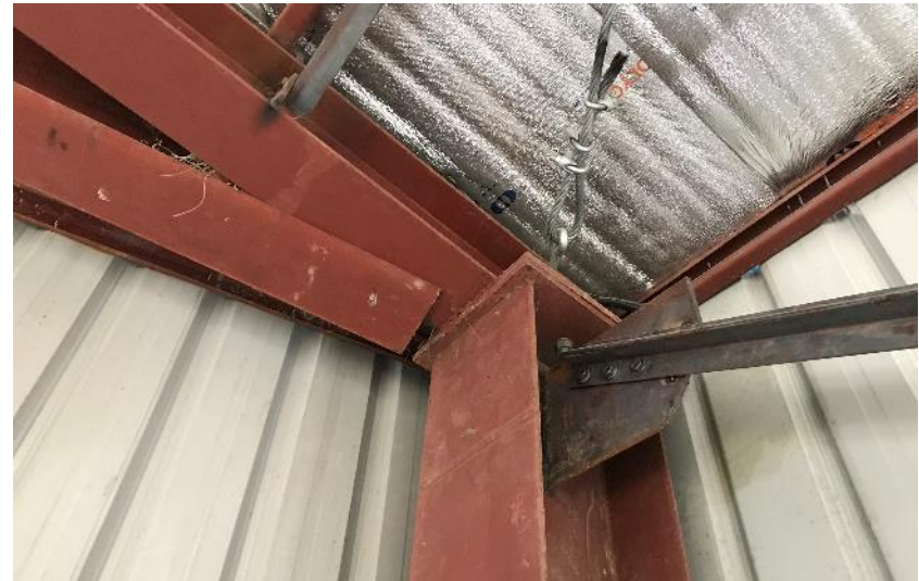
Improper connection observed at rafter and column joint.
