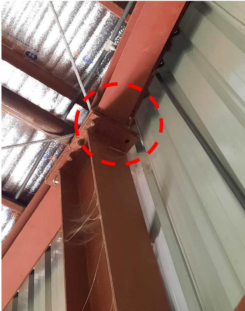
Missing bolts in the connection
