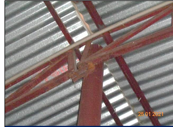
Poor connection details
