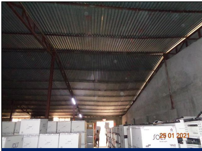
Purlin was found sagging
