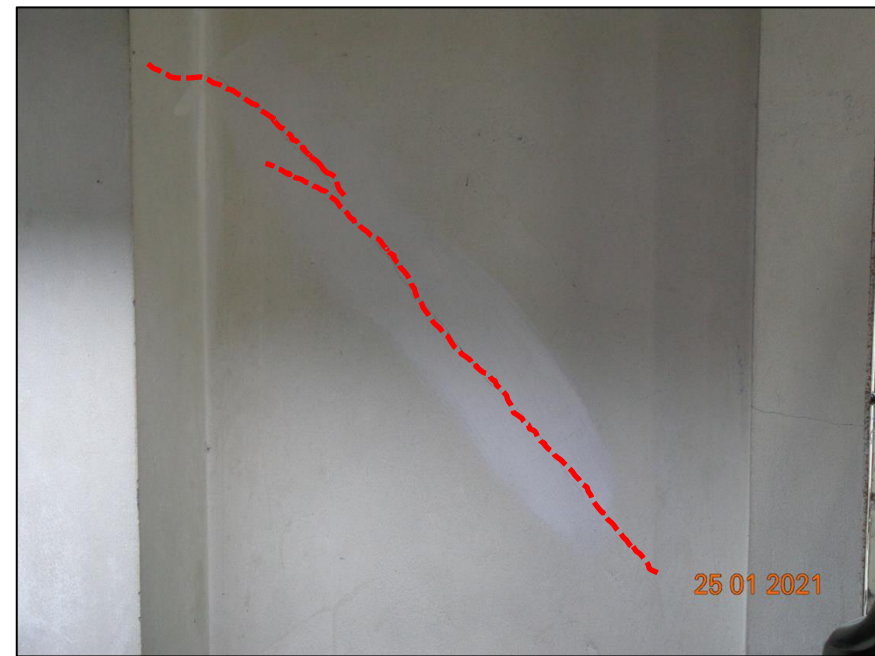
Crack in brick wall
