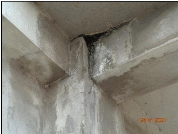
Dampness in Beam & Column
