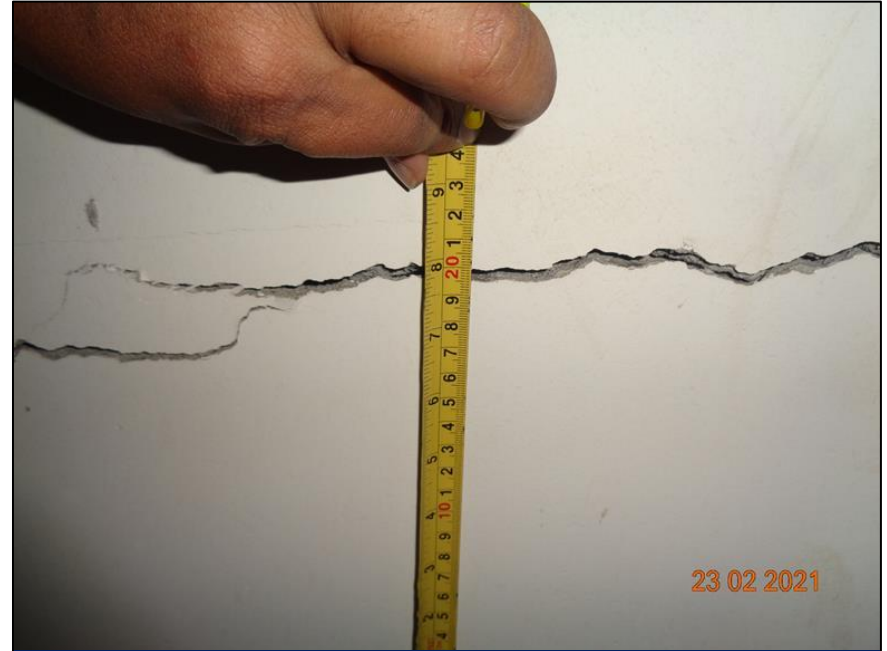
Thickness of crack
