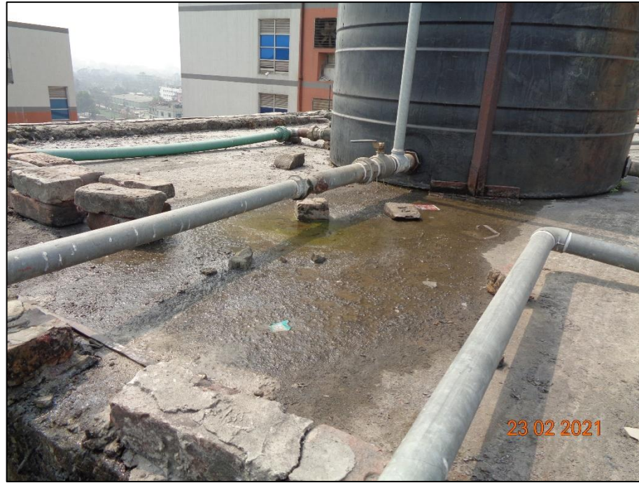
Water leakage at roof & stair roof
