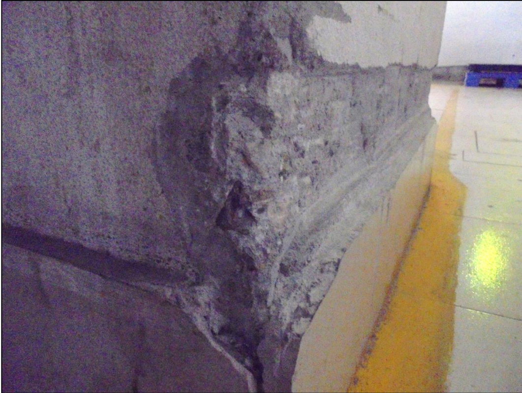
Damage column at 5 th floor
