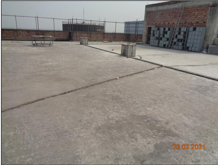
No water proofing layer
