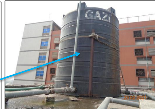
Undocumented water tank
