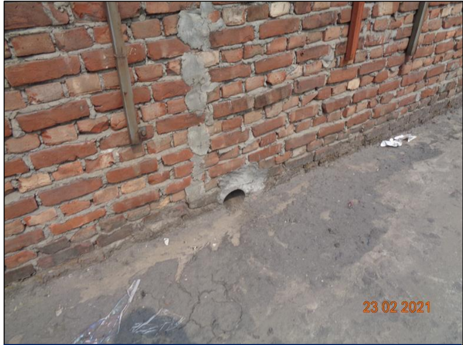
Signage of water clogging
