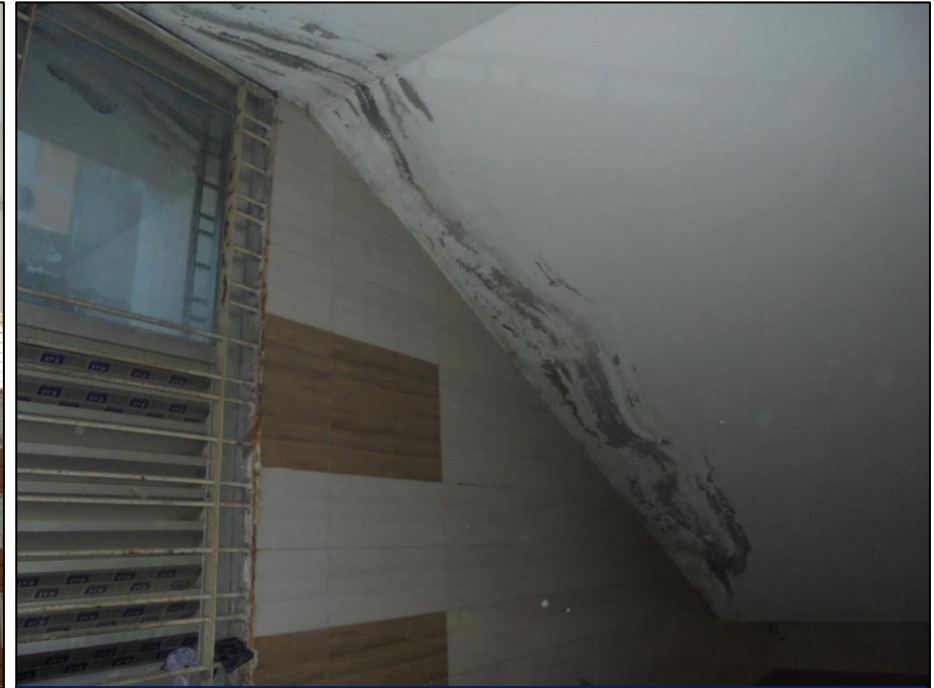
Dampness in stair bottom slab
