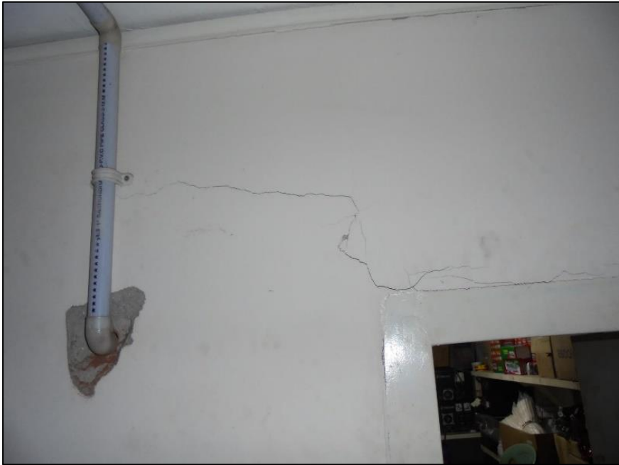
Crack in brick wall
