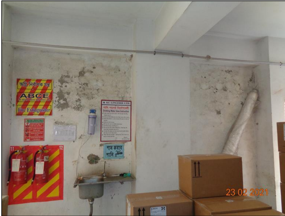
Dampness in periphery brick wall at 5 th floor
