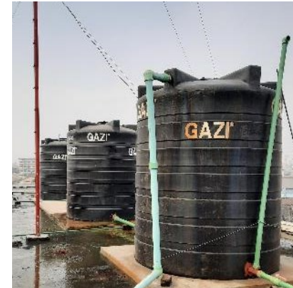
10000 liters water tank source of heavy loading
