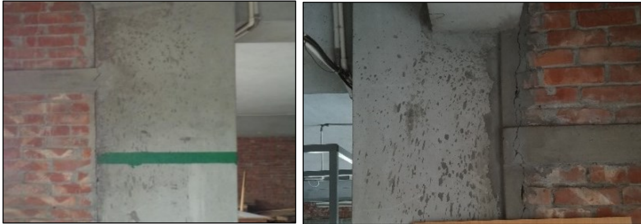
Cracks between columns and wall connection
