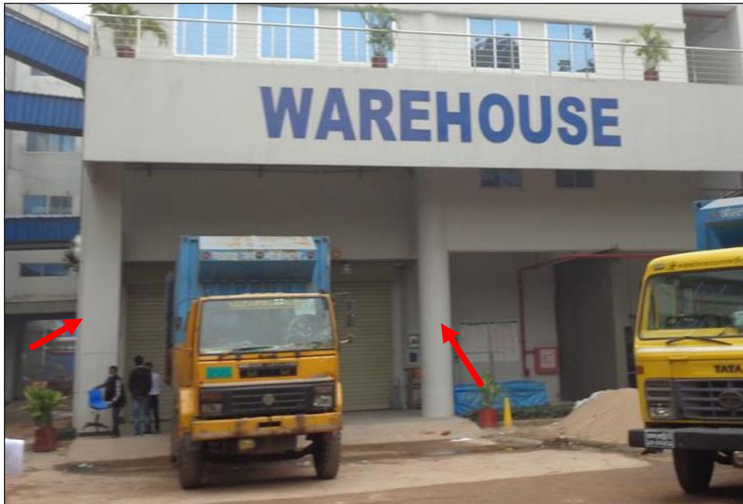
Column susceptible to vehicle impact
