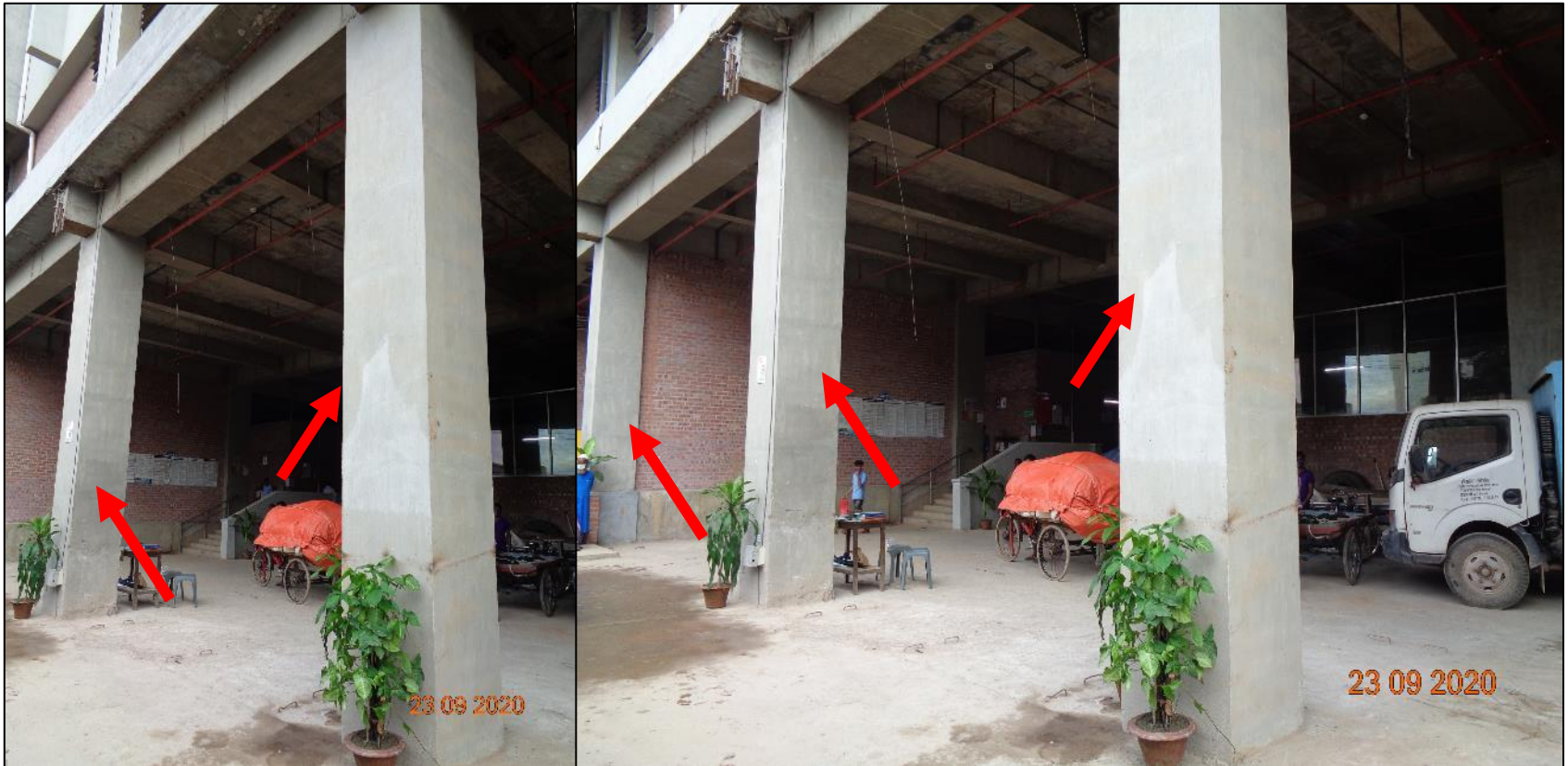
Column susceptible to vehicle impact
