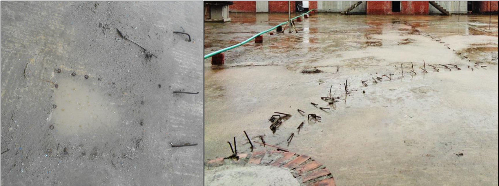
Exposed re-bar at roof
