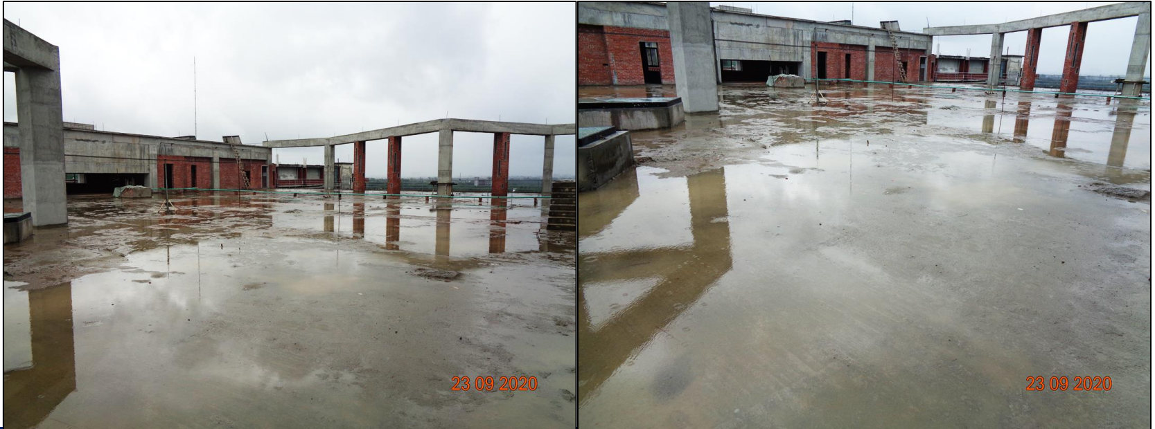
Lack of water proofing & water ponding
