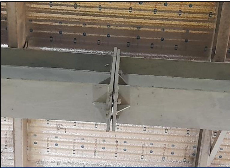
Significant connection gap
