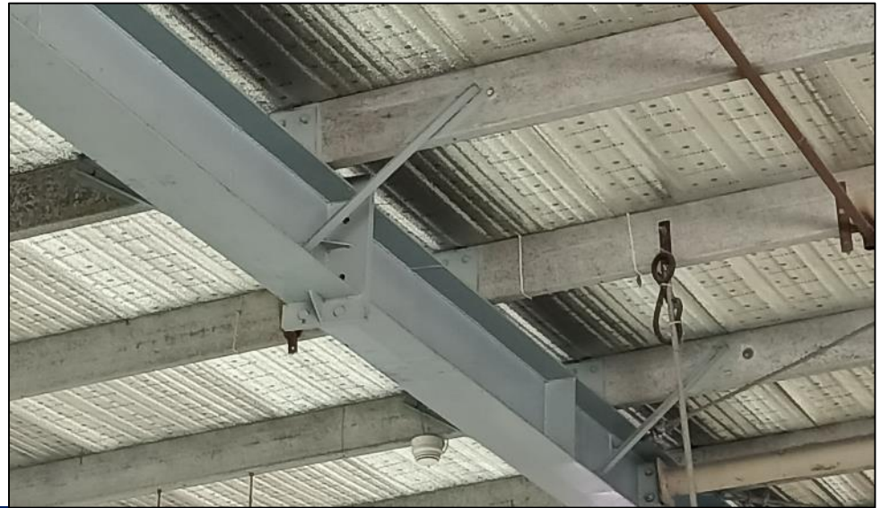
Bolt missing at several locations
