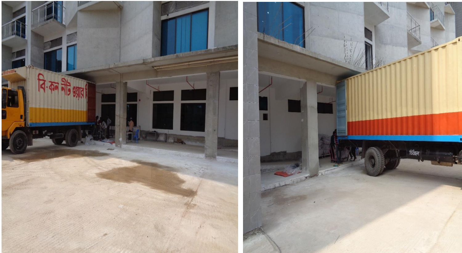
Columns prone to possible vehicle impact
