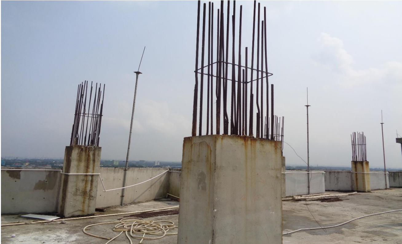
Exposed reinforcement left at roof level
