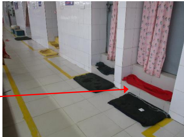
Approx. 450 mm floor rise on ground to 3rd floor and 200 mm on other floors
