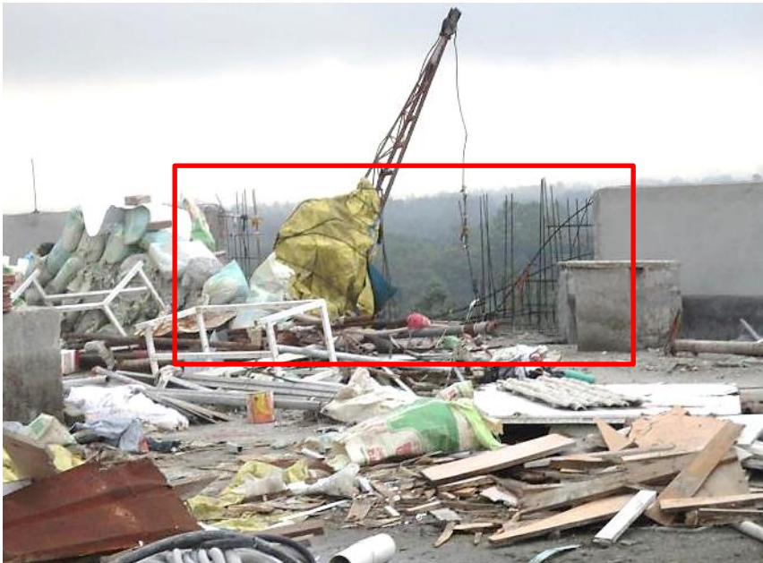
Roof parapet wall missing on the eastern side
