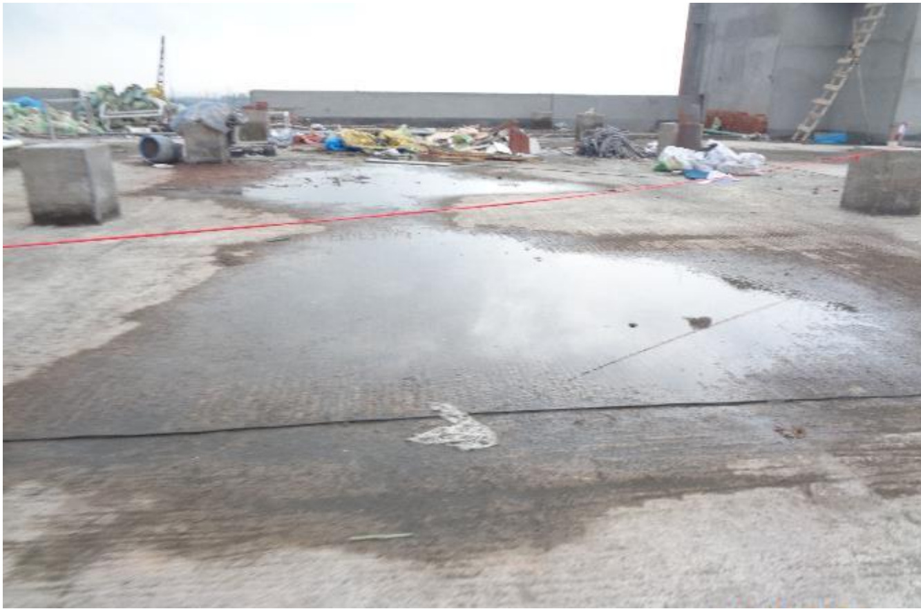
Stagnant water observed on roof
