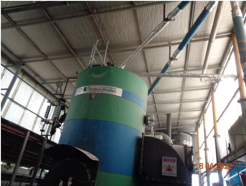
Inside of Jhut Boiler
