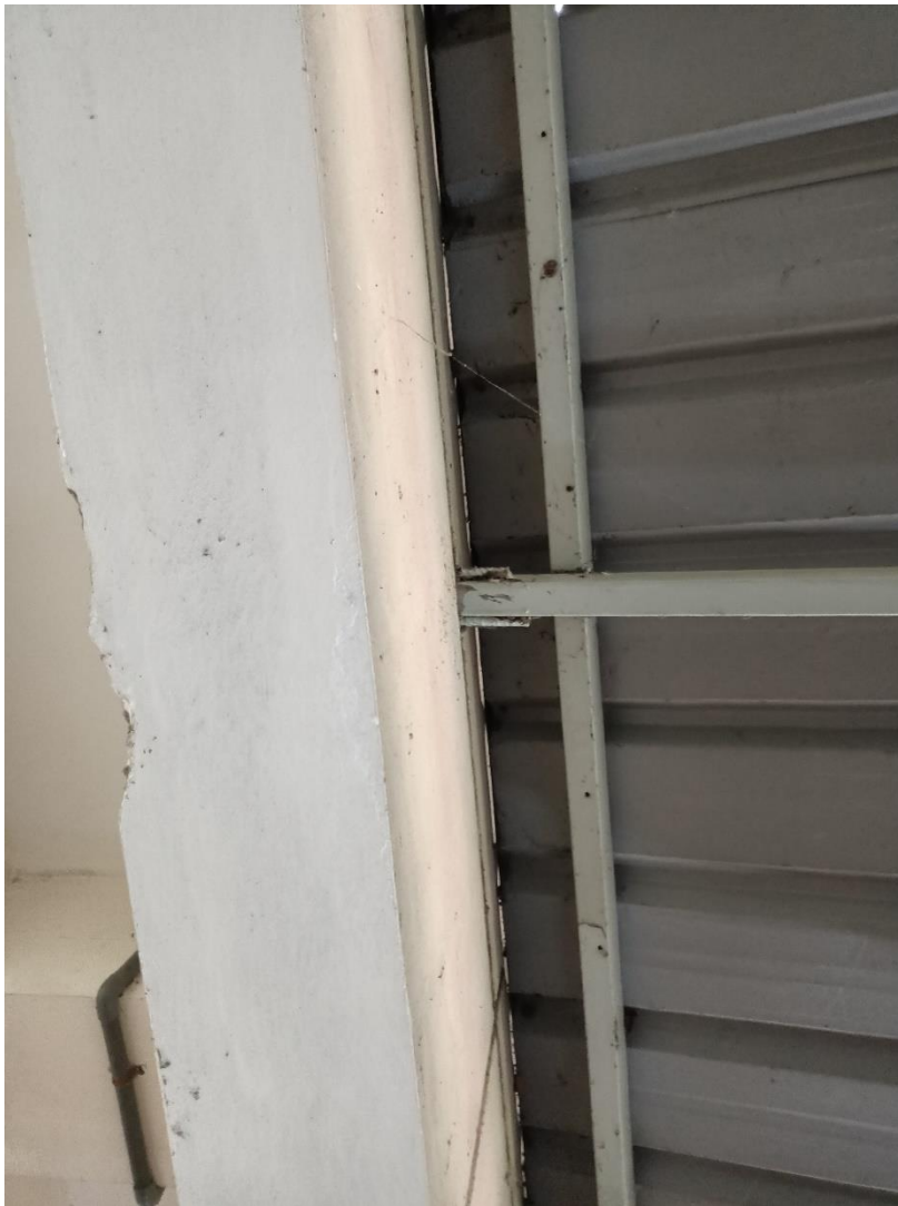
Apparently inadequate connection
