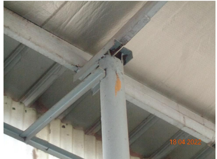
Non engineered connection
