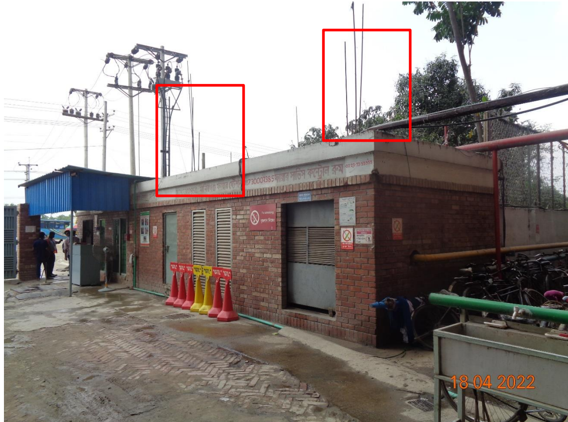
Exposed rebar at column on the roof
