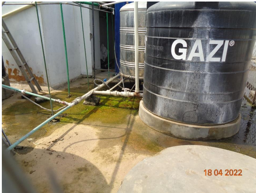
Plastic water tank on roof
