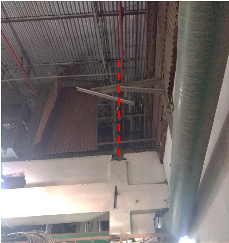
Truss found as out of plumb (Steel part)
