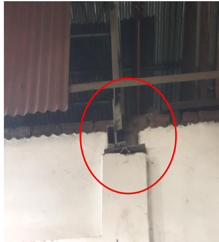
Poor connection between truss and RC column (Steel part)
