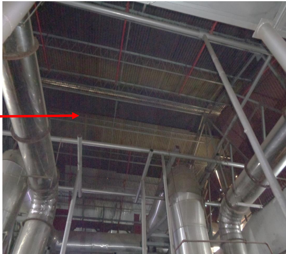
Roof bracing is not provided (Generator part)
