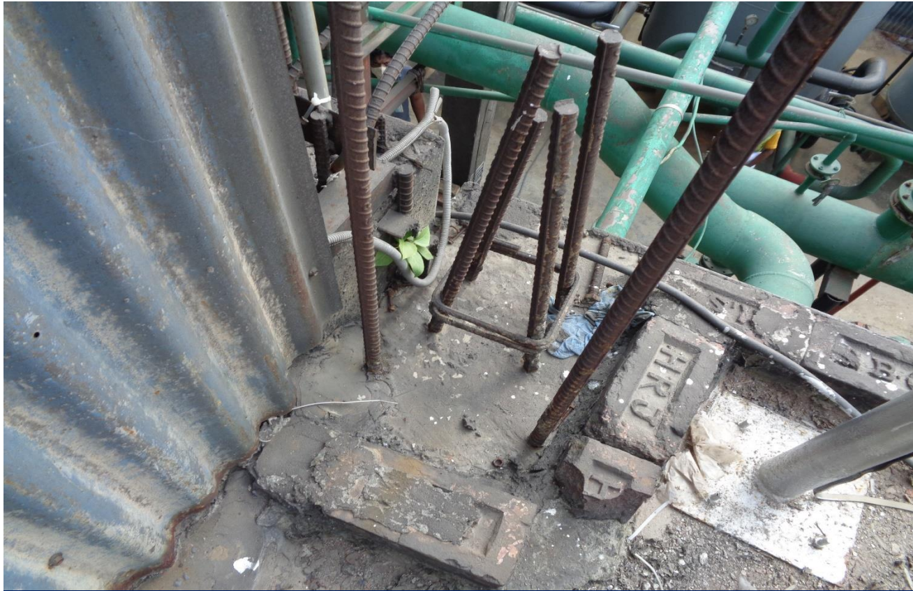
Exposed rebar at roof level (RC part)
