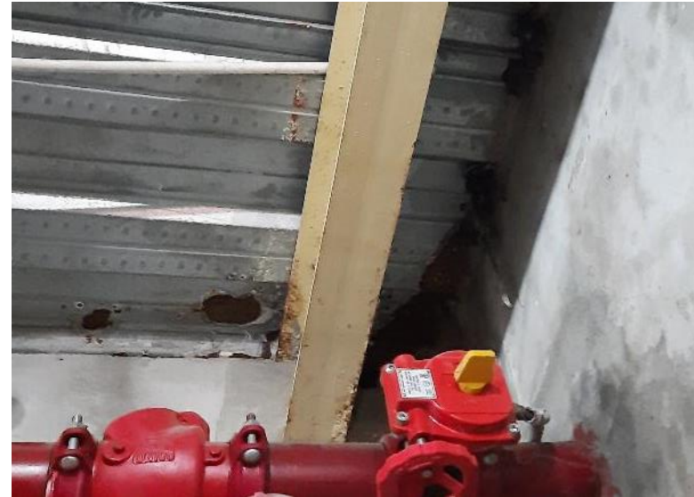
Corrosion in sub-beam
