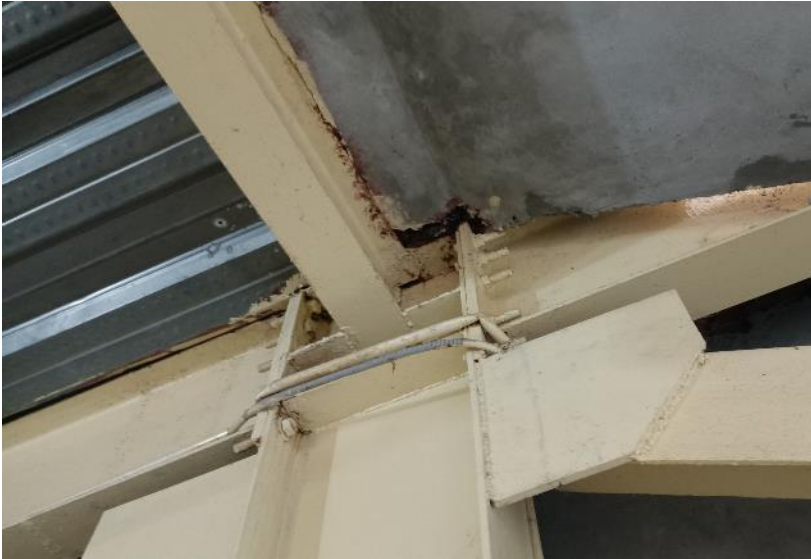
Corrosion in joint
