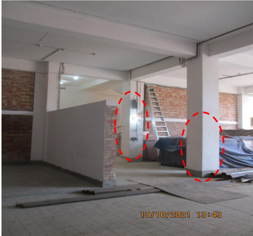
Column susceptible to vehicle impact
