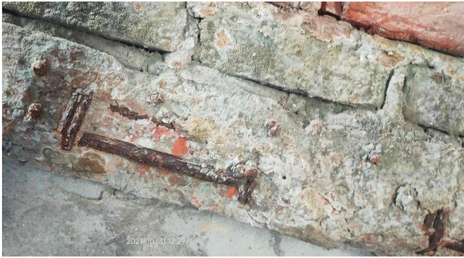
Corrosion of slab rebar
