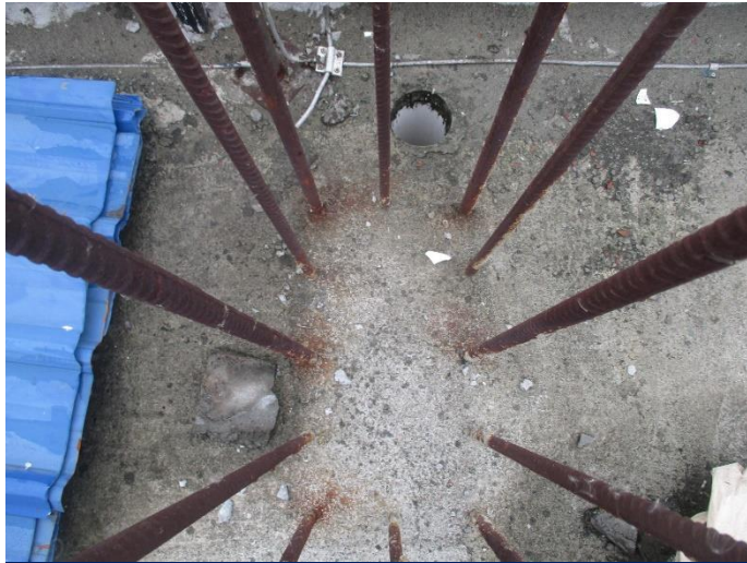
B-14: Exposed rebar on roof
