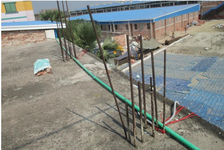
B-8: Exposed rebar on roof
