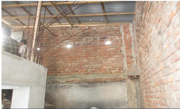
Beam missing on roof
