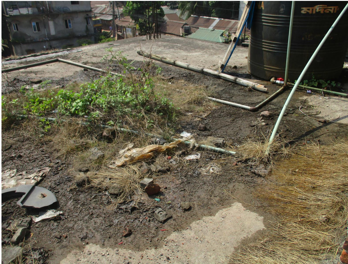
Water ponding and vegetation on roof
