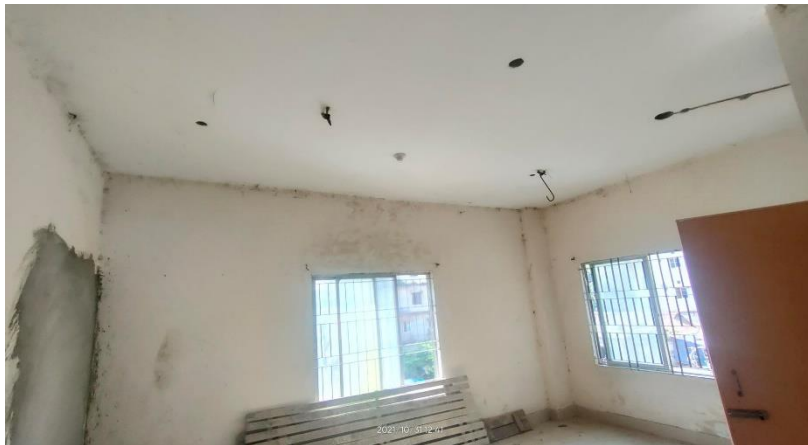
Beam missing on 1st floor roof
