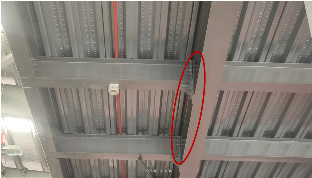
Gap between steel joints
