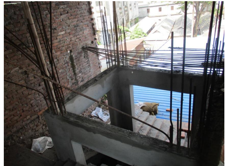
Exposed rebar on roof and stair zone
