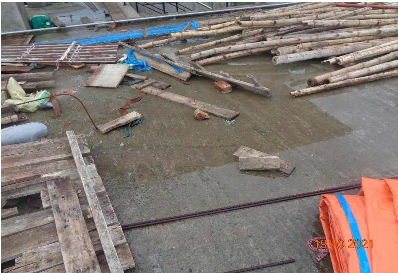
Stagnant water observed on roof
