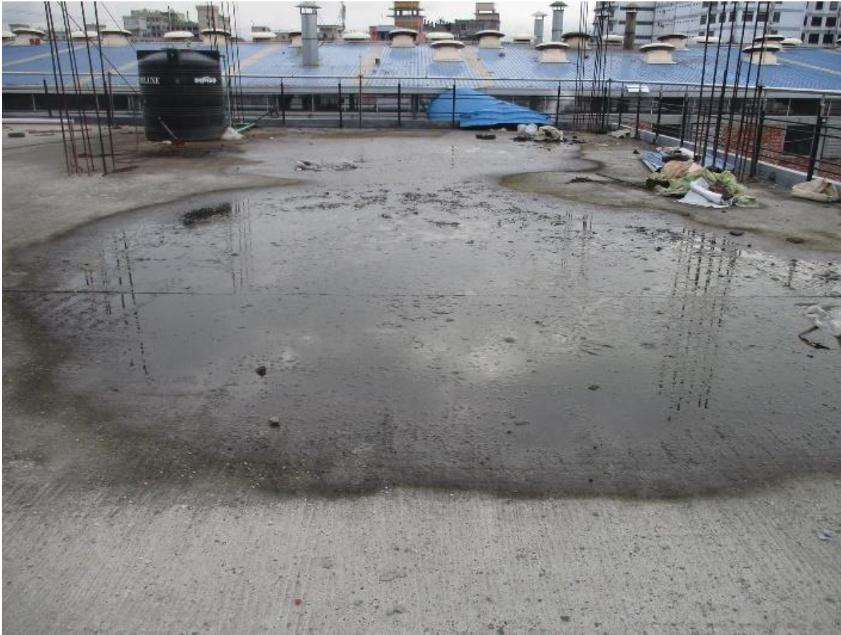
Water ponding on roof
