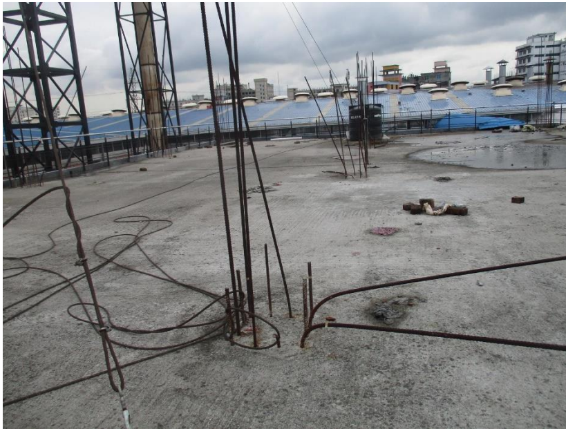
Exposed rebar on roof
