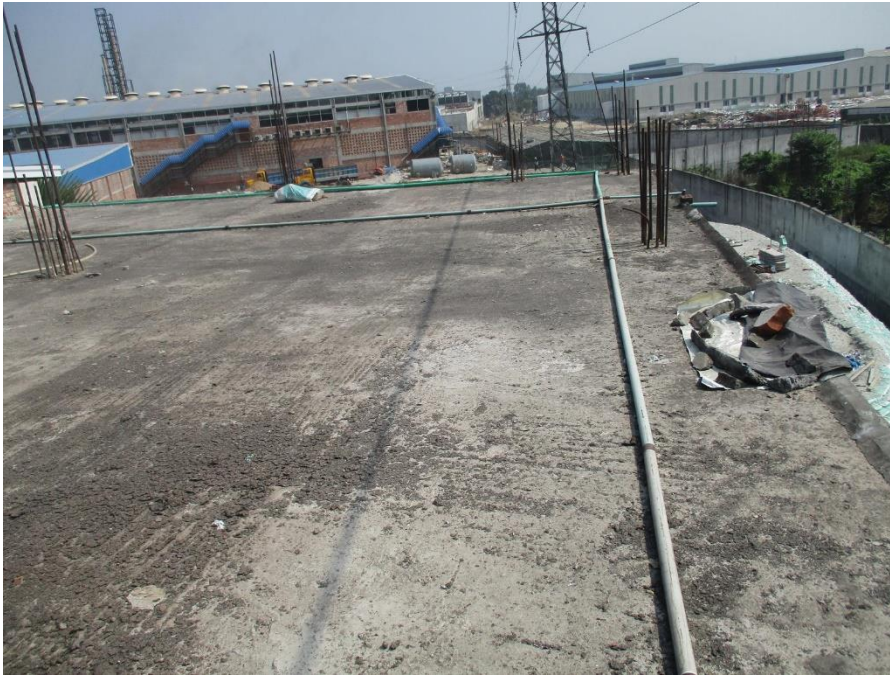
No parapet/barrier on roof
