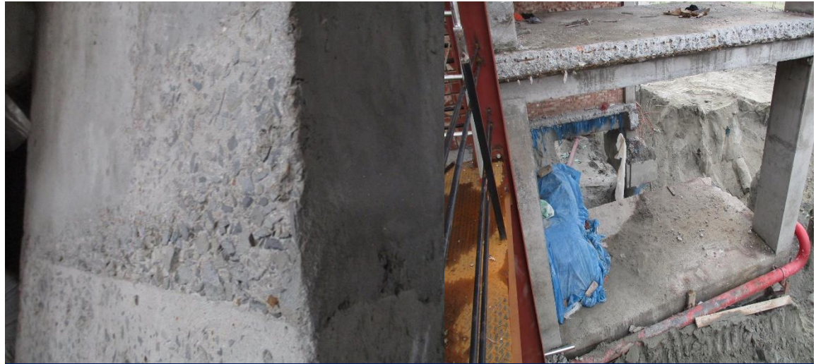
B-14: Stone aggregate on column and slab
