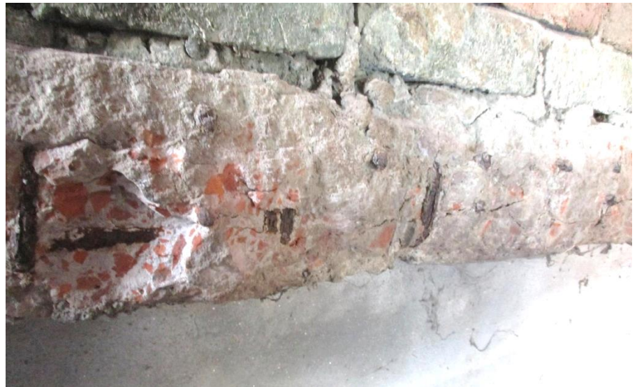
Spalling of concrete
