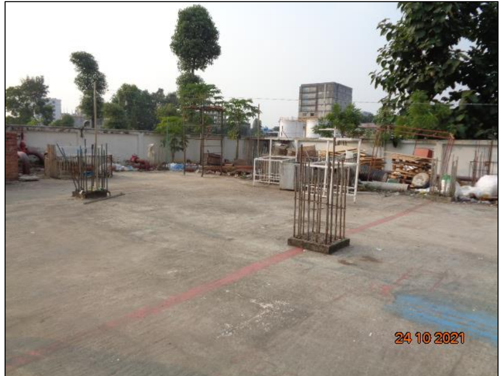
Exposed rebar at ground floor
