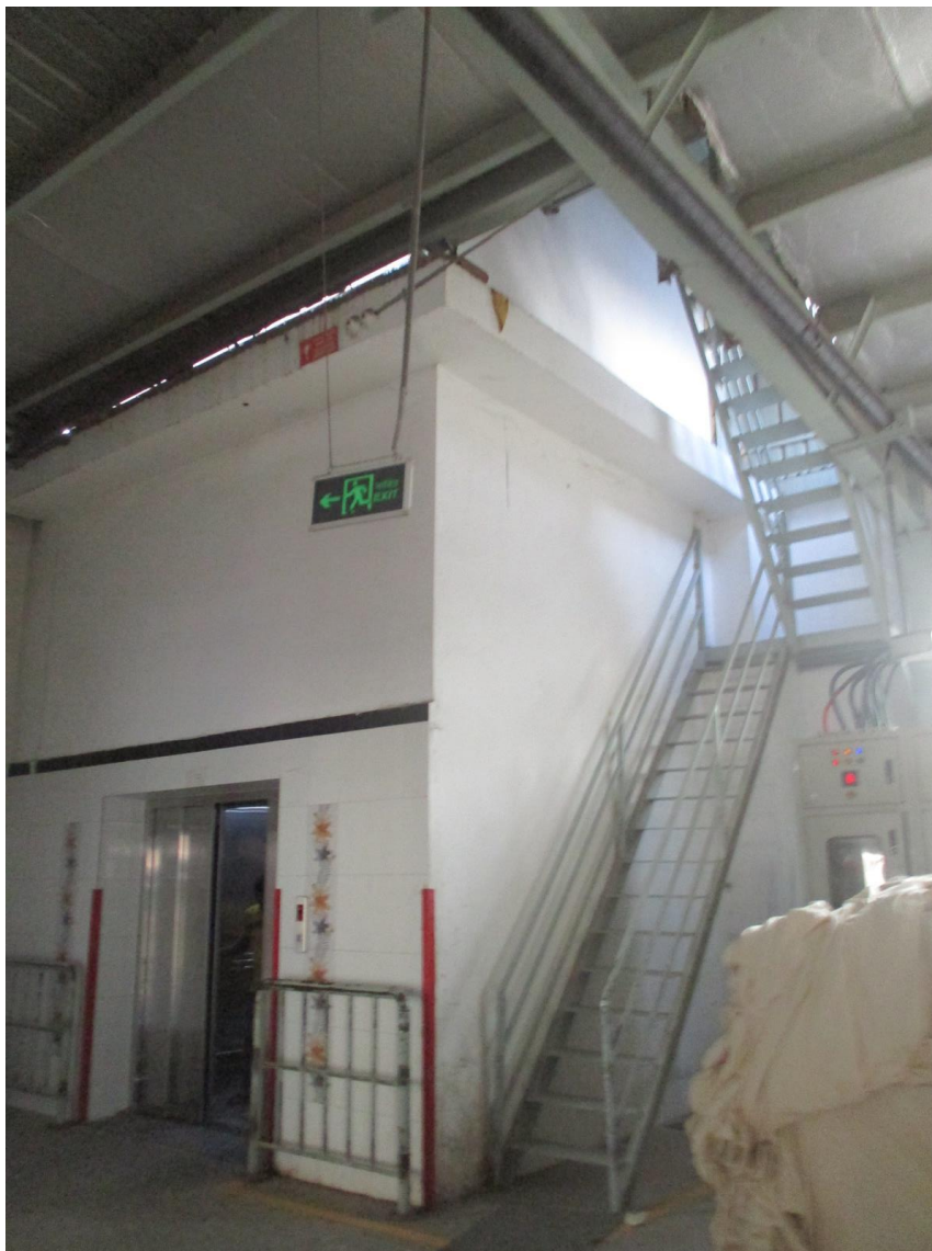
Steel stair from 1st floor to lift machine room
