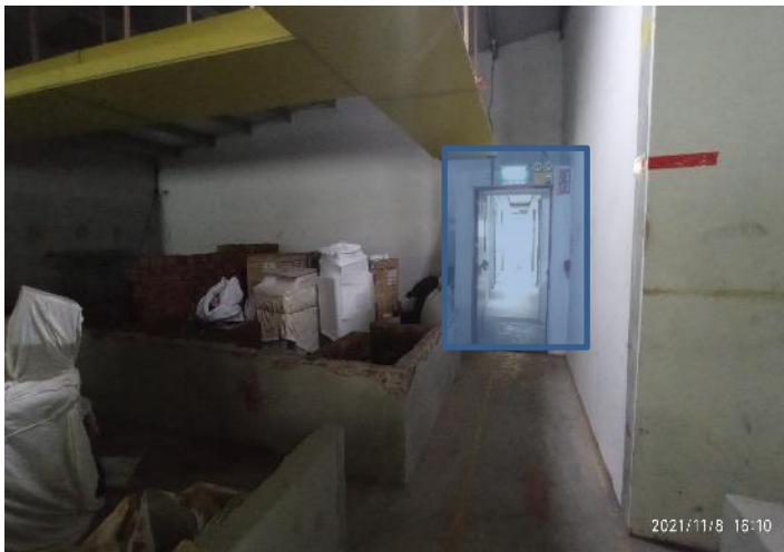
Mismatch in wall layout at 1F (Fire door wall)
