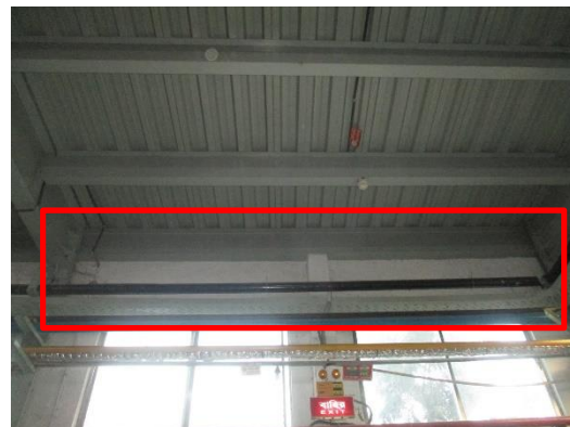
Beam MB-2 found on-site instead of RMB-2
