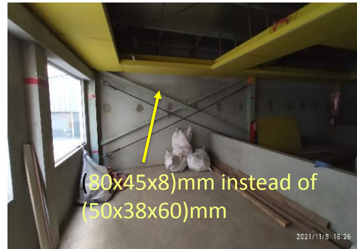
Mismatch in C-Channel bracing size
