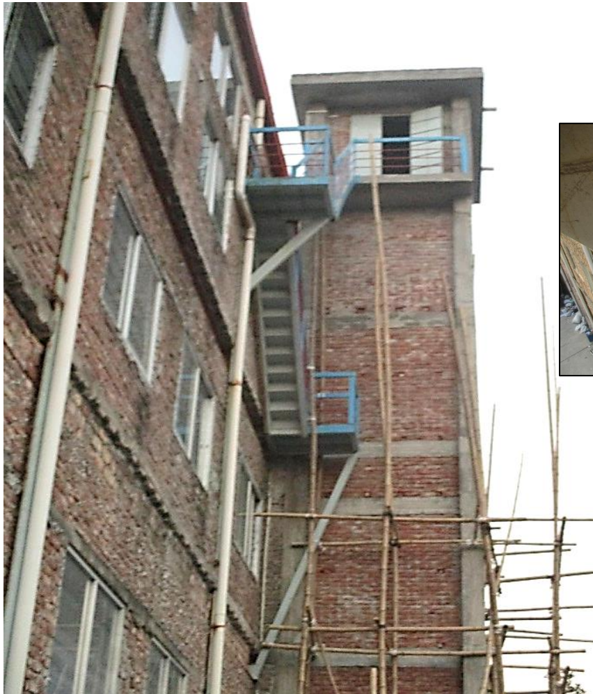
Steel stair from 1st floor to lift machine room
