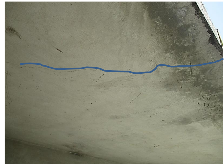
Hairline crack on the slab soffit
