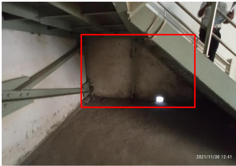
Missing bracing in stair
