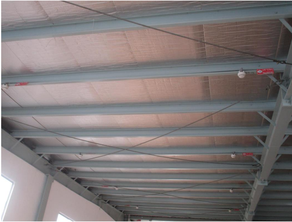
Loose cable bracing
